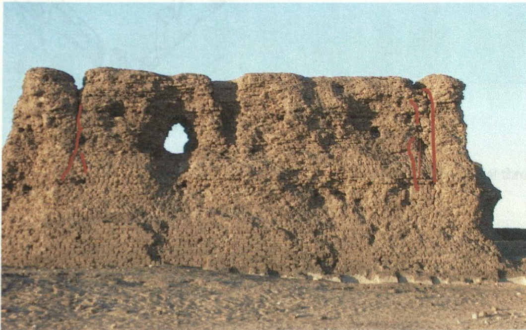
Figure 48: East side of the north section of the east wall showing the pattern of cracks at the ends of high walls.
