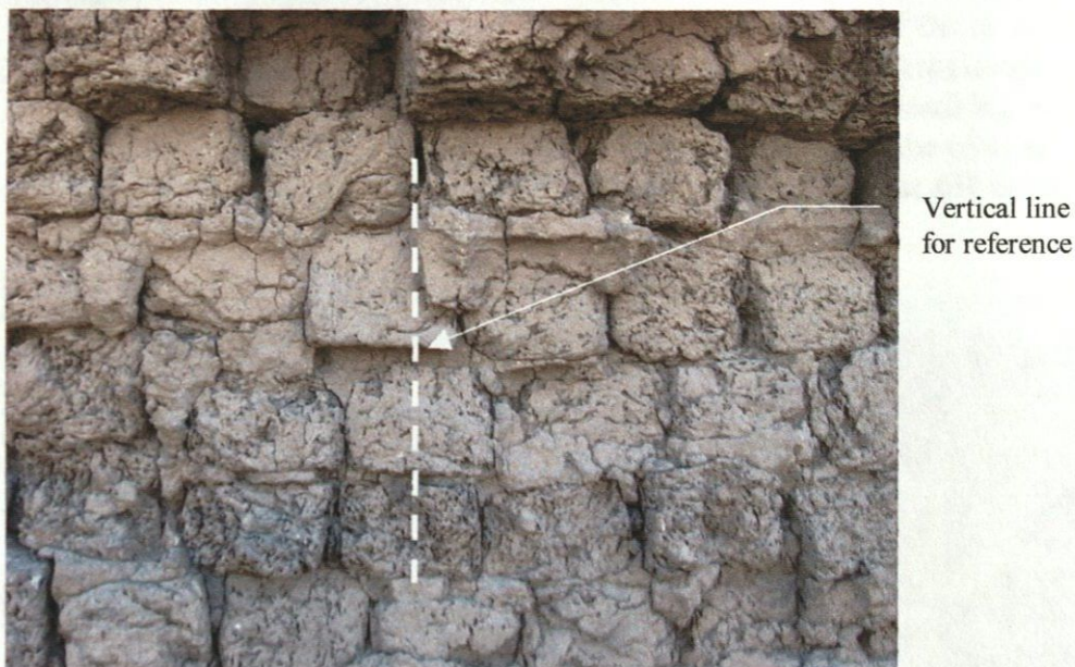
Figure 15: Detail of a typical wall showing through-wall headers and occurrence of stacked joints.
