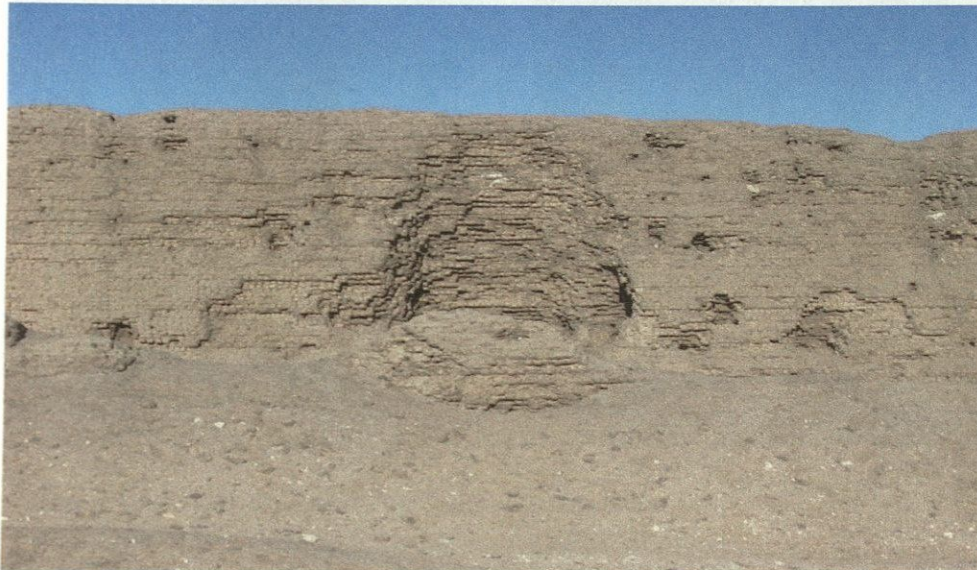
Figure 4: A detail of the west side of the west wall showing the visual impact of one of the Coptic cells cut into the wall.
