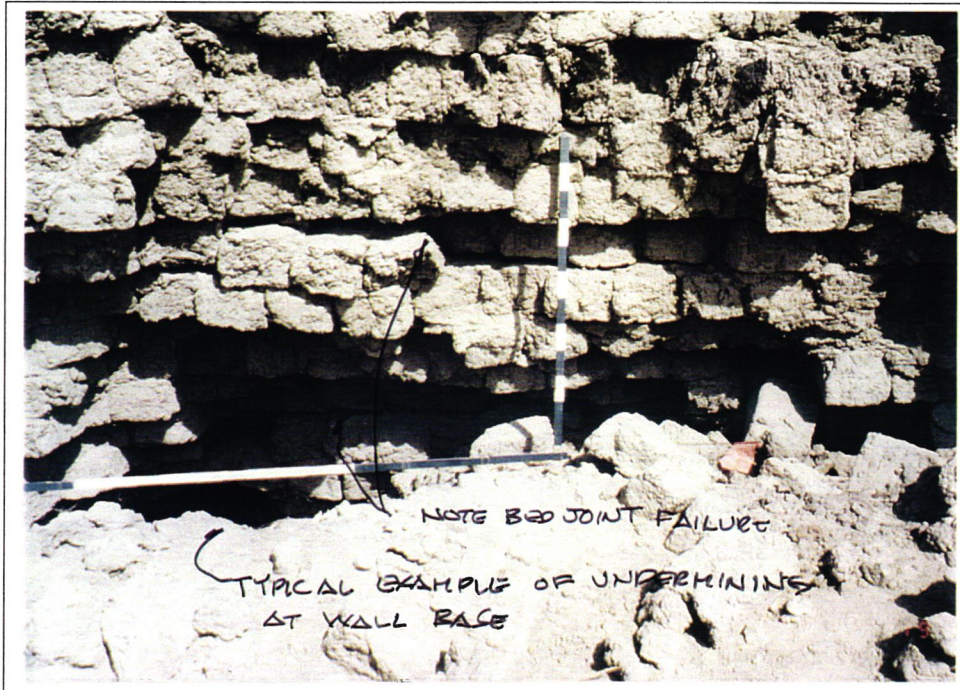
Photograph No. 49 Undermining at East Main Enclosure Wall
