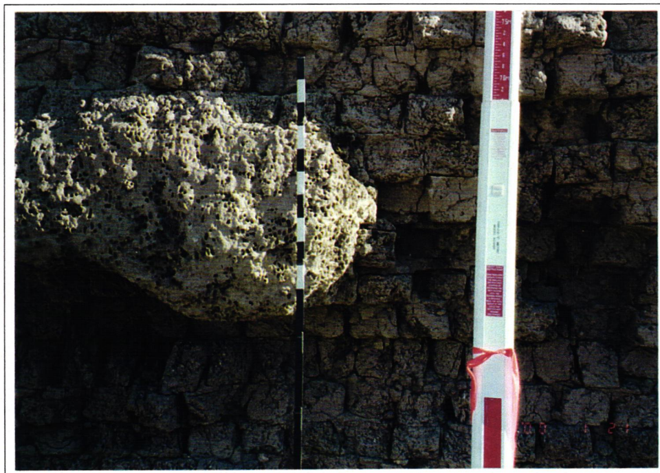
Photograph No. 26 Mud Wasp Accretion
