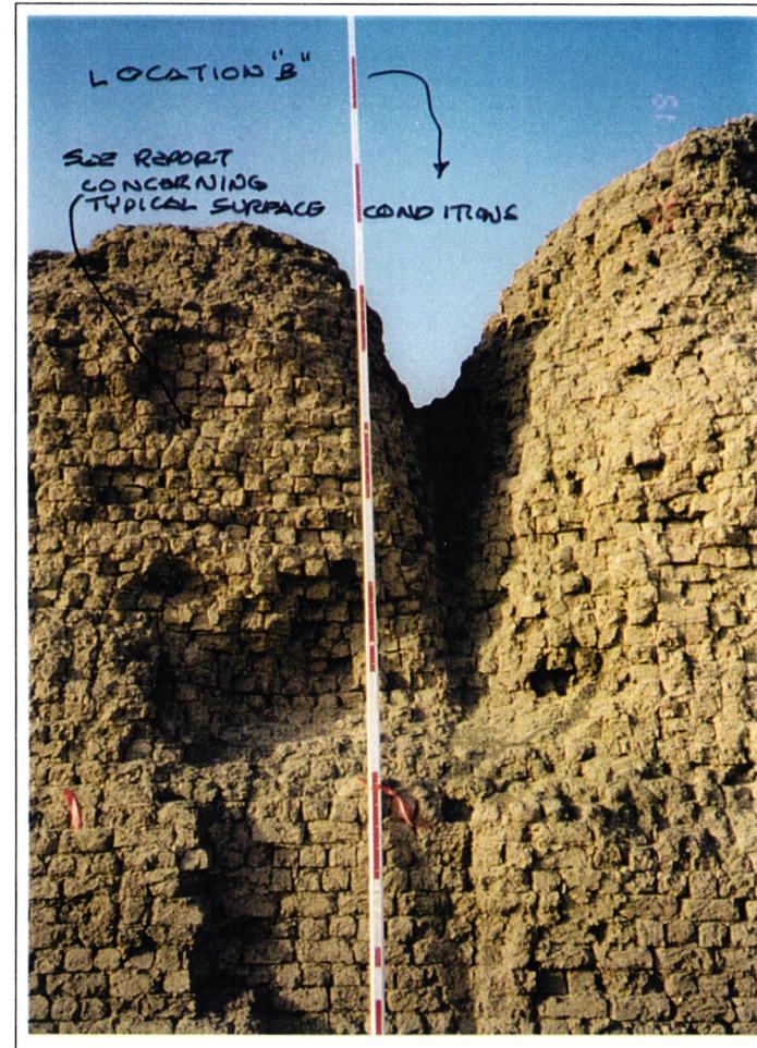
Photograph No. 38 Erosion at Location "B"
