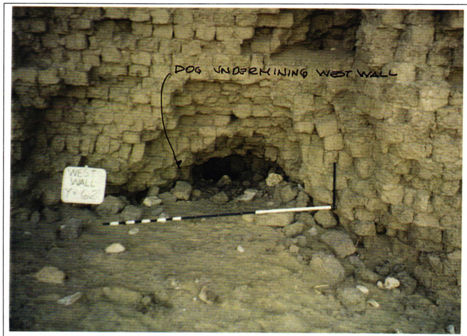
Photograph No. 22 Base Undermining
