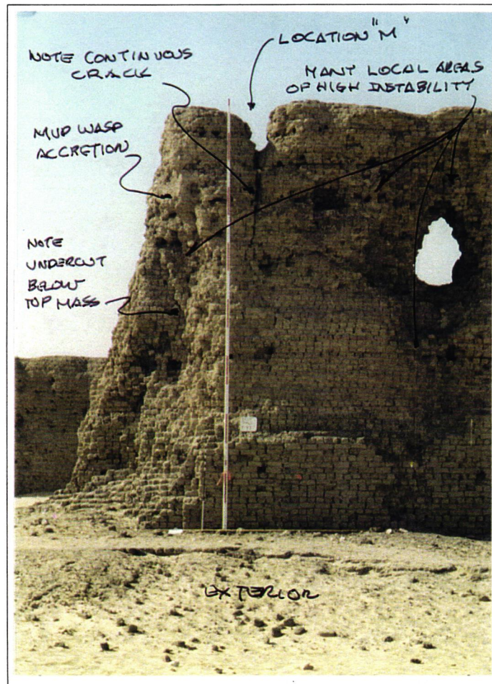
Photograph No. 58 Cracking at South End of "Section 4"
