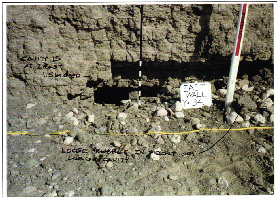
Photograph No. 20 Base Undermining
