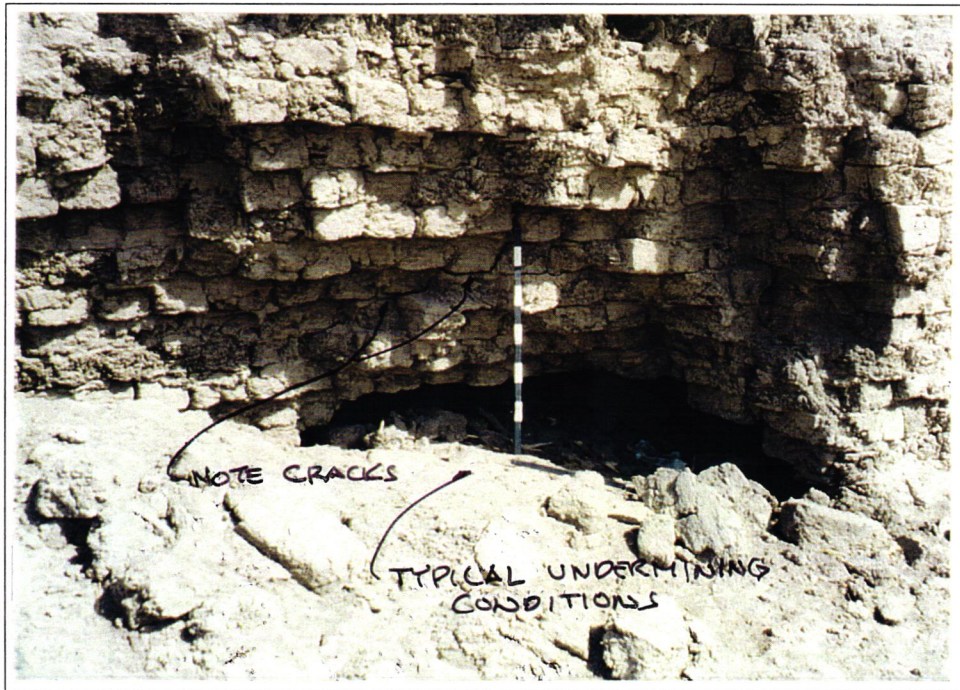
Photograph No. 50 Undermining at East Main Enclosure Wall
