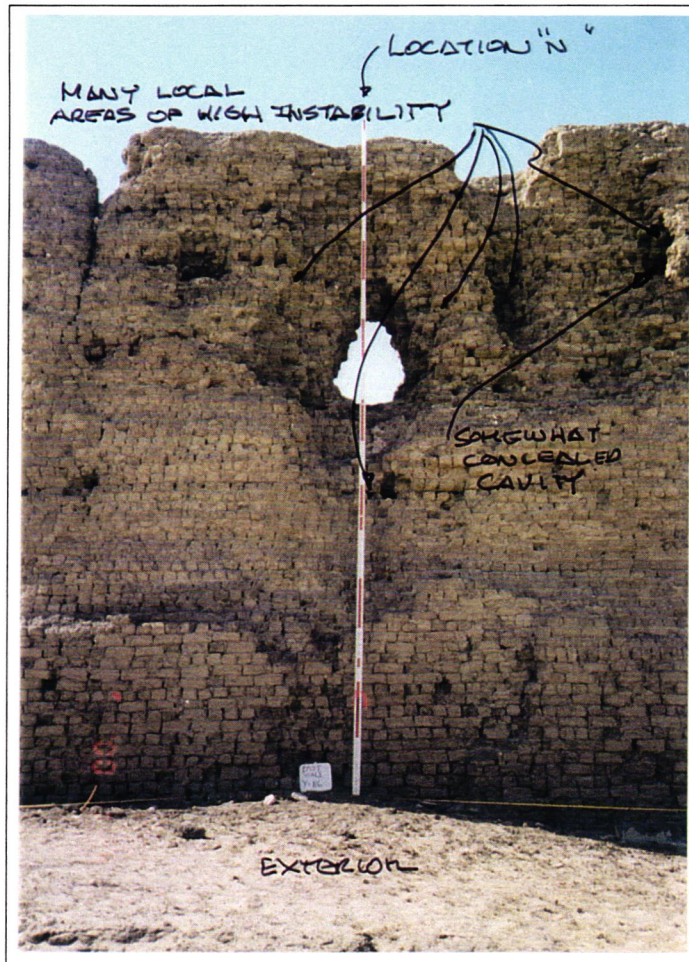
Photograph No. 61 "Section 4" Deficiencies at Location "N"
