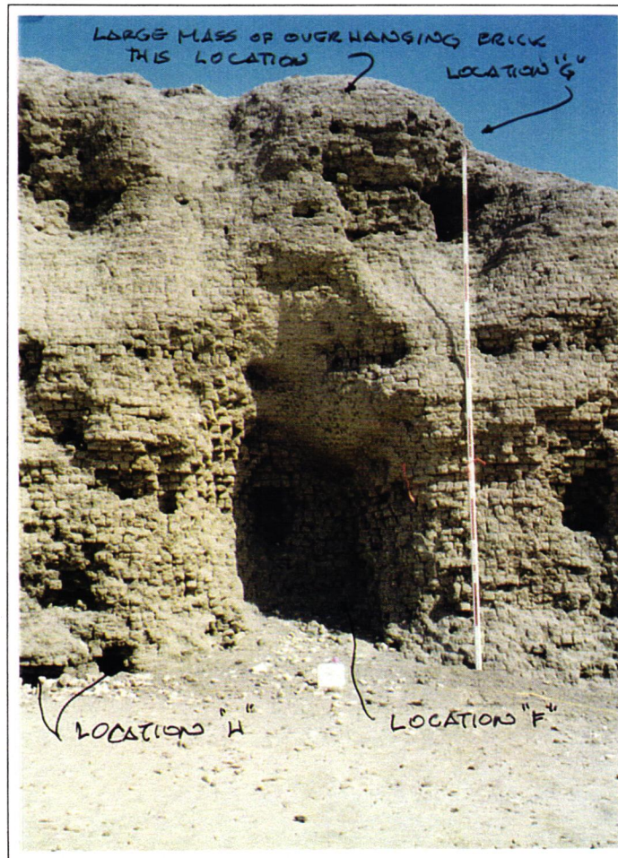
Photograph No. 40 Location "F" and "G" East Main Enclosure Wall Interior View
