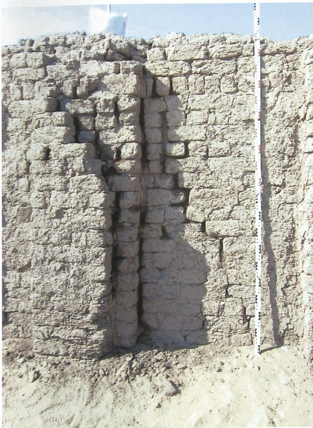
Figure 10: Pilaster on east elevation of East Enclosure Wall that was stabilized by repointing and grouting in March 2001. The dark mortar joints are still damp.
