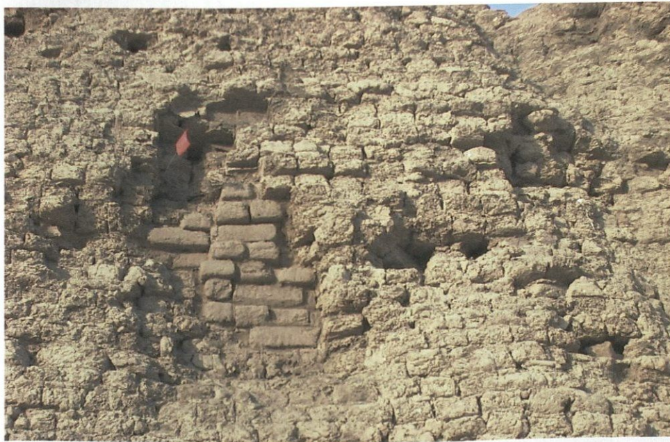
Figure 6: Detail of the void repair in the West Enclosure Wall. The new mud bricks are stepped to support the unsupported mud bricks above, and set to replicate the characteristic of the surrounding mud brick wall.
