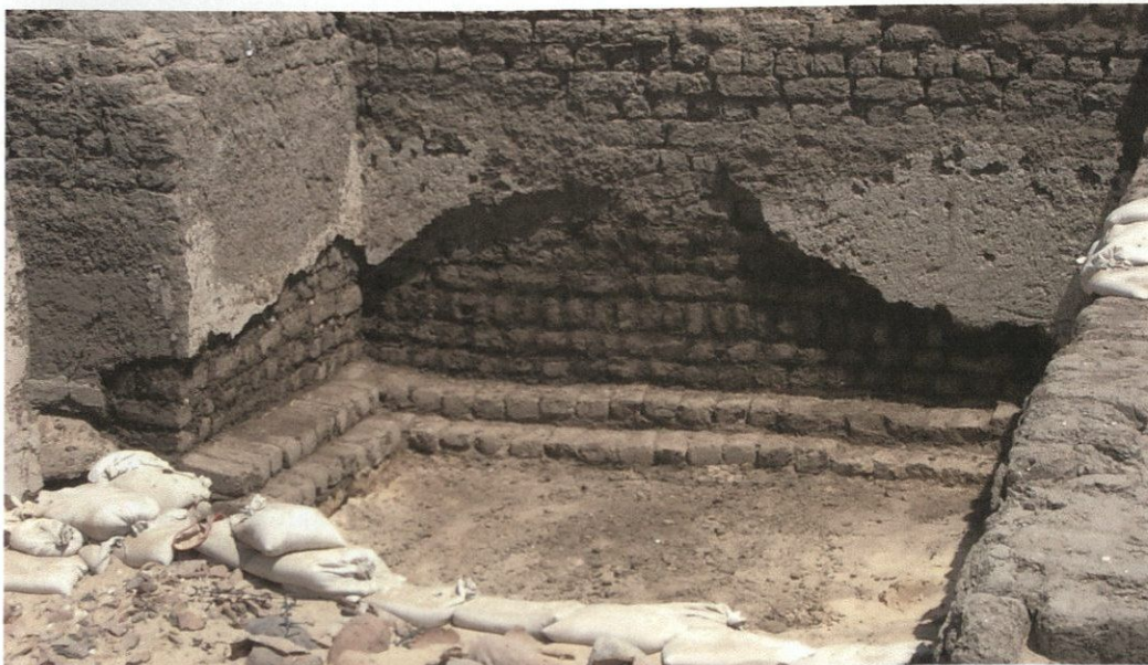
Figure 11: The completed construction of a wall base. The lower part of the wall will be covered with fill sand.
