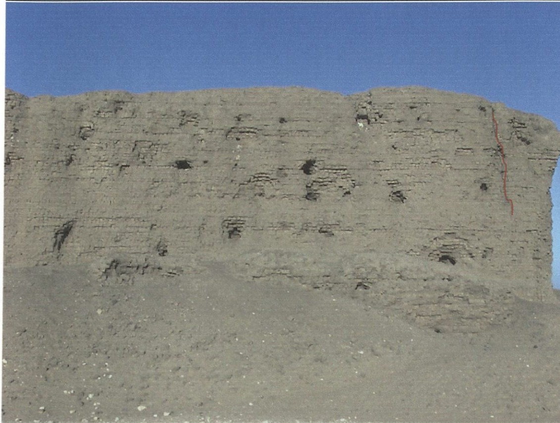
Figure 1: West Enclosure Wall with a major structural crack near the end of the wall. These type cracks are common near the ends of the tall walls.
