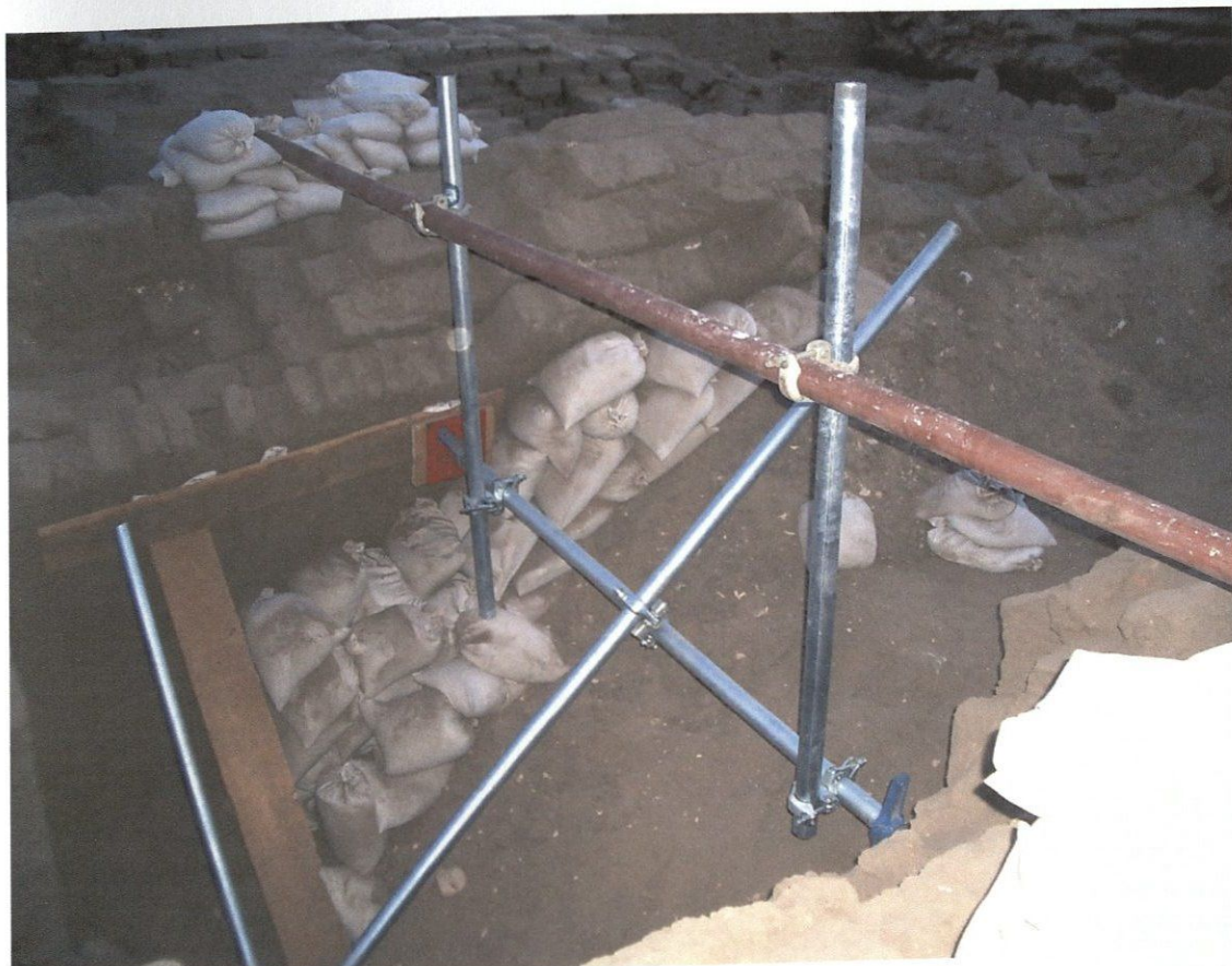
Figure 5: one brace or one bay of the system installed. Additional bays can be added as needed as the excavation continues. Note that the system is supported from above leaving the floor clear for continuing the excavations.
