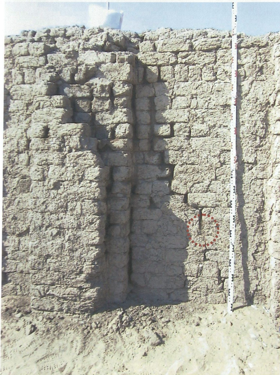
Figure 5: Cracks filled on a rear of the east elevation of the East Enclosure Wall that will serve as the approved panel for similar work. This is the same area as Figure 3. See Figure 6 for a detail of the area in red.
