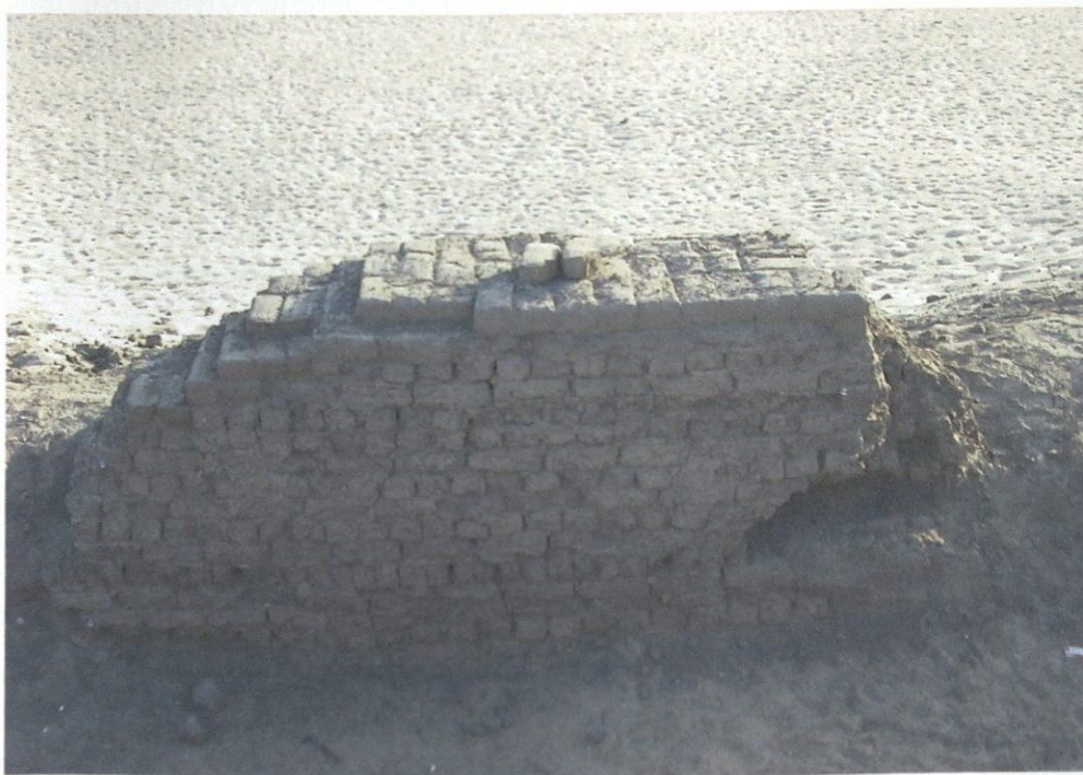
Figure 4: The same low East Perimeter Wall after the cap was constructed in March 2001.
