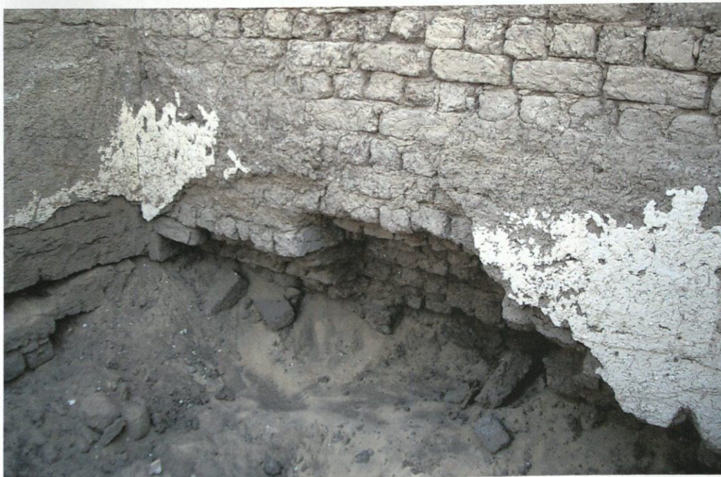
Figure 1: Base of wall that has collapsed and will have to be reconstructed to provide structural integrity.
