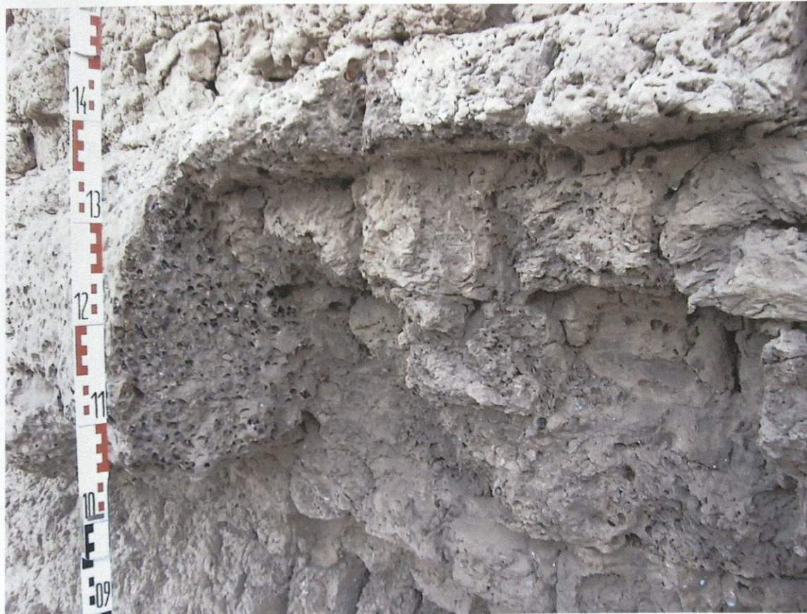
Figure 3: A detail of the area where the insect nest was removed
