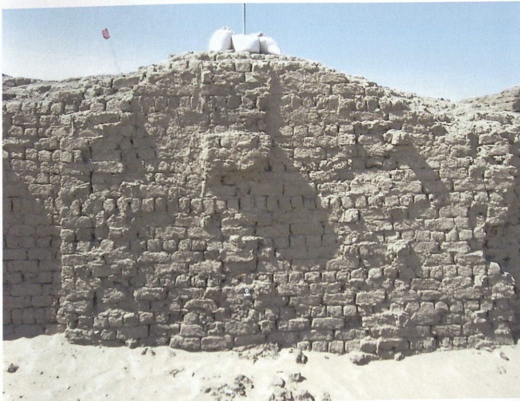
Figure 1: An area on the East Enclosure Wall showing three deteriorated pilasters.
