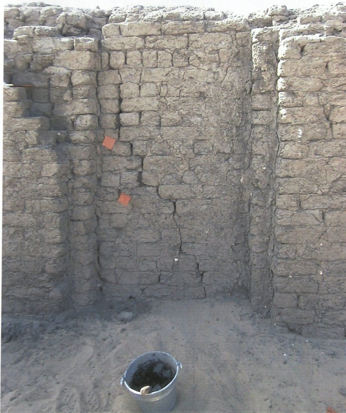
Figure 3: Detail of the East Enclosure Wall showing numerous cracks that are structurally related to the critical condition on the opposite side of the wall.
