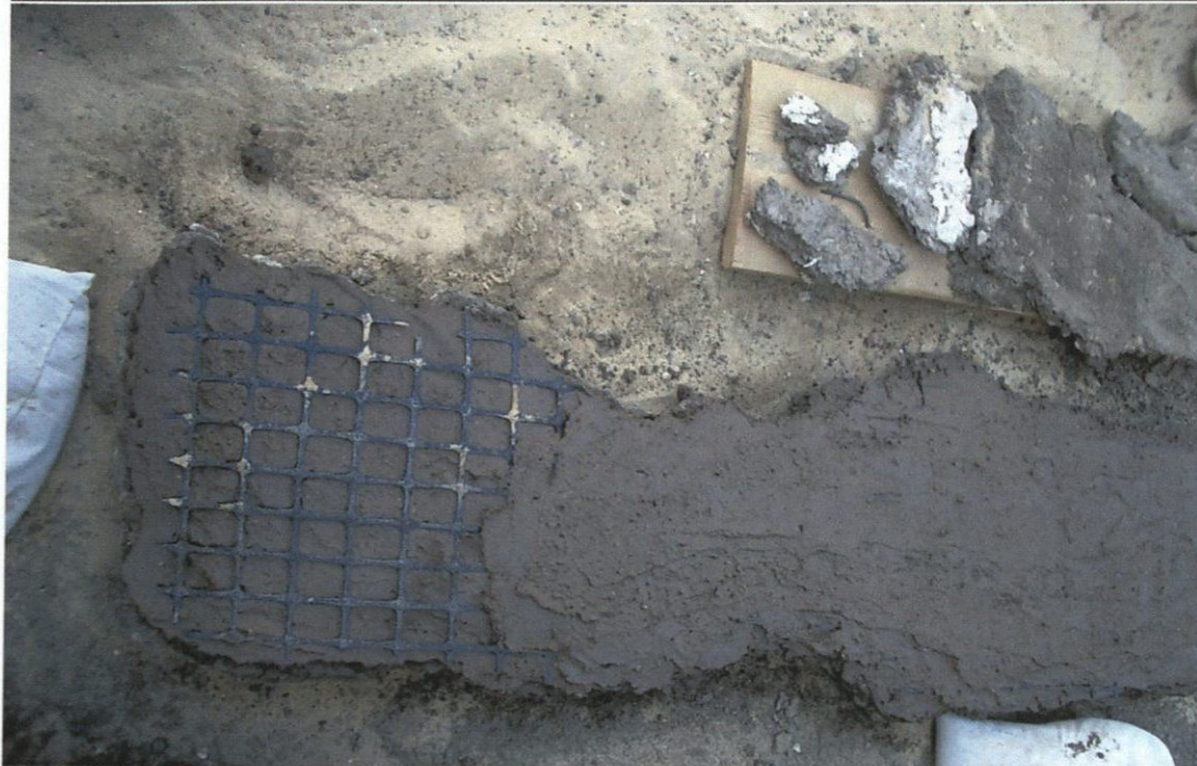
Figure 6: Detached plaster with geogrid being attached to the back with mud plaster.
