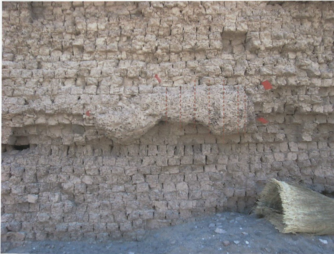
Figure 1: A large insect nest on the lower part of the north side of the South Enclosure Wall prior to the removal that is specified in this section. The red dotted vertical lines are the approximate locations of the chisel cuts into the nest.
