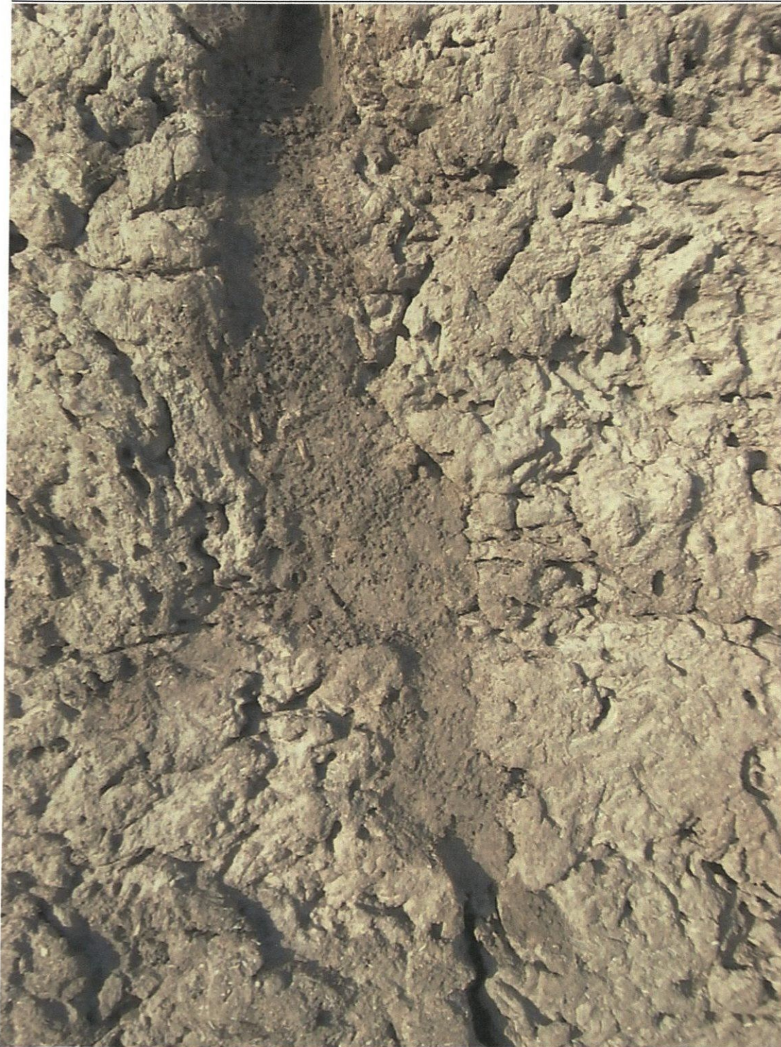
Figure 6: Detail of the wall shown in Figure 5 showing a detail of the approved technique for minor crack repair. Note that the still-damp mortar has been textured with a stiff bristle brush to blend better with the original material.
