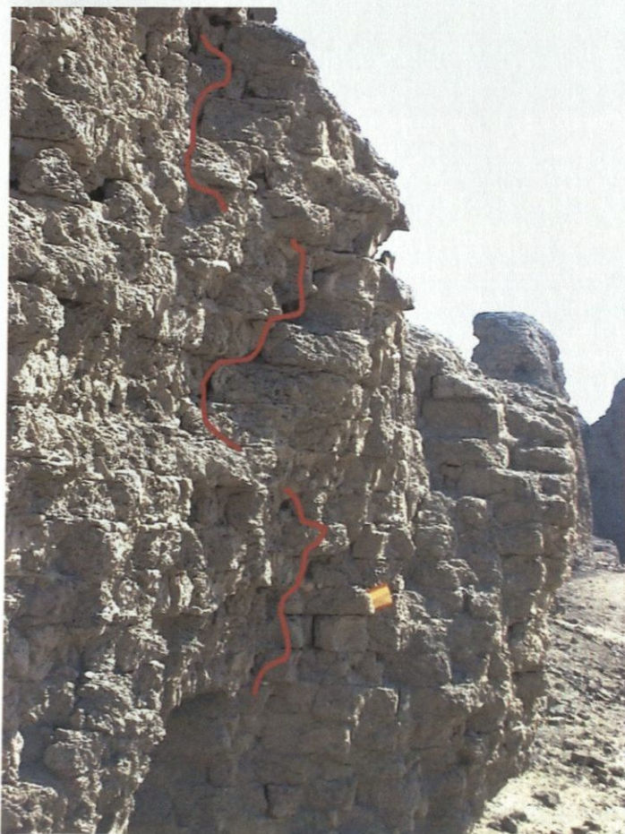
Figure 1: Detail of crack in the East Enclosure Wall. This is a large structural crack that will require grouting because of the depth of the crack.
