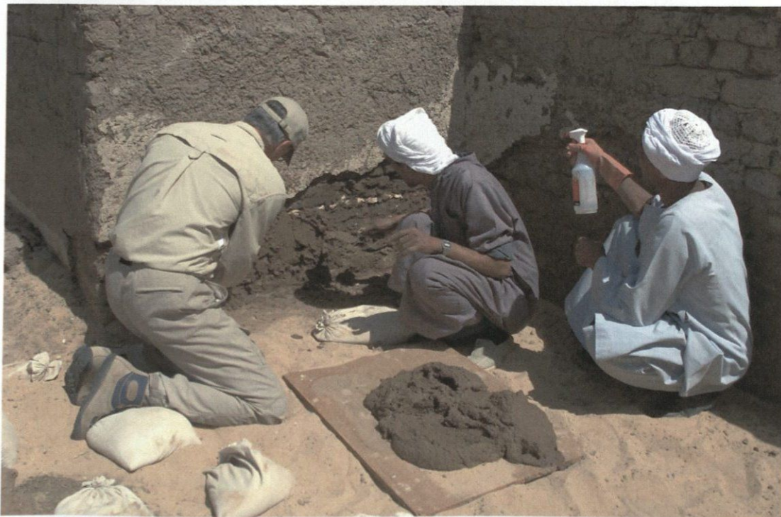
Figure 7: Mud plaster being applied to mud brick substrate for reattaching the plaster.
