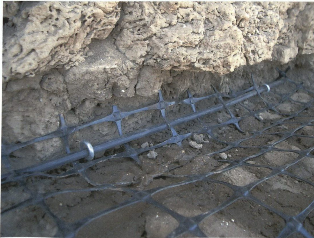
Figure 6: Mechanical ties used to connect horizontal reinforcement and new mud brick construction to existing.
