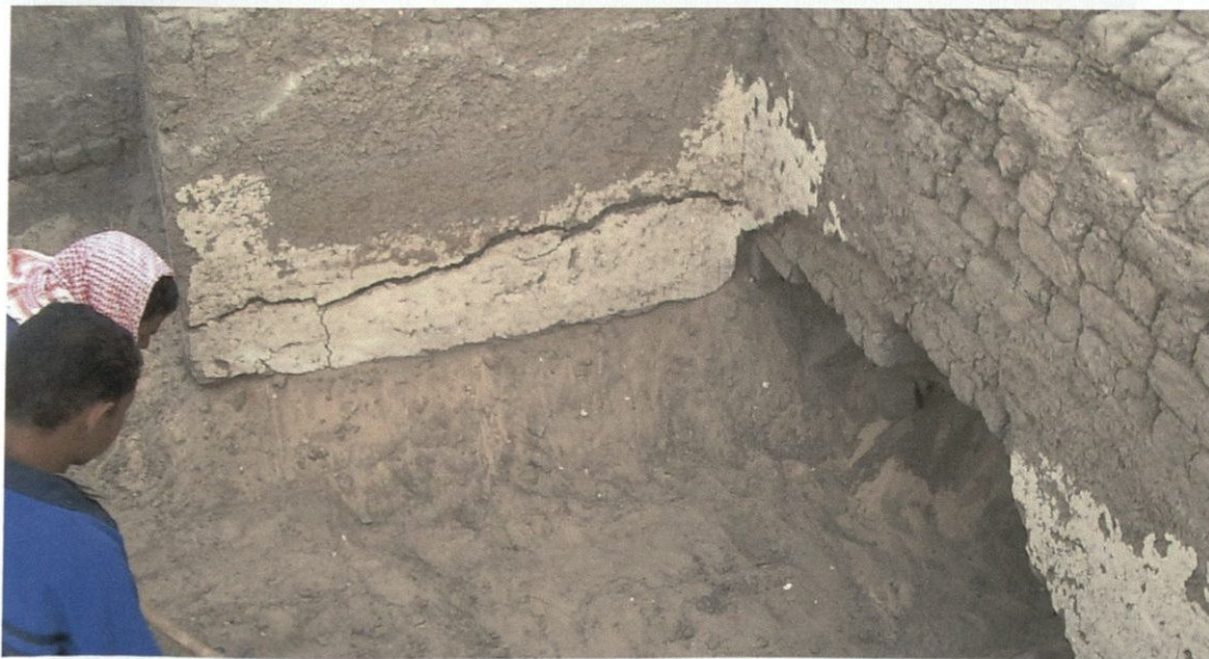
Figure 3: Detached plaster prior to removal from wall.
