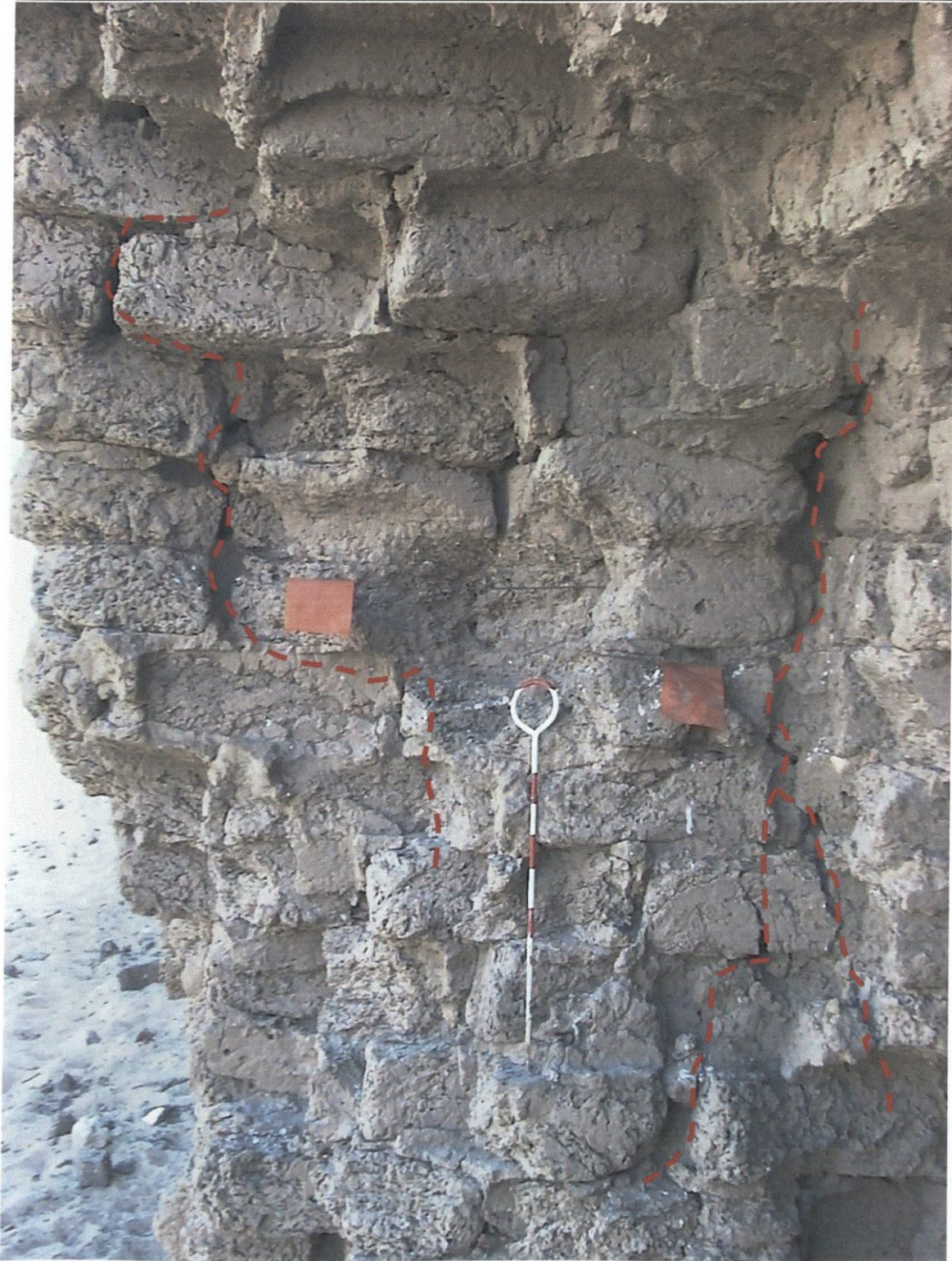
Figure 2: A detail of the West Enclosure Wall showing numerous smaller cracks.
