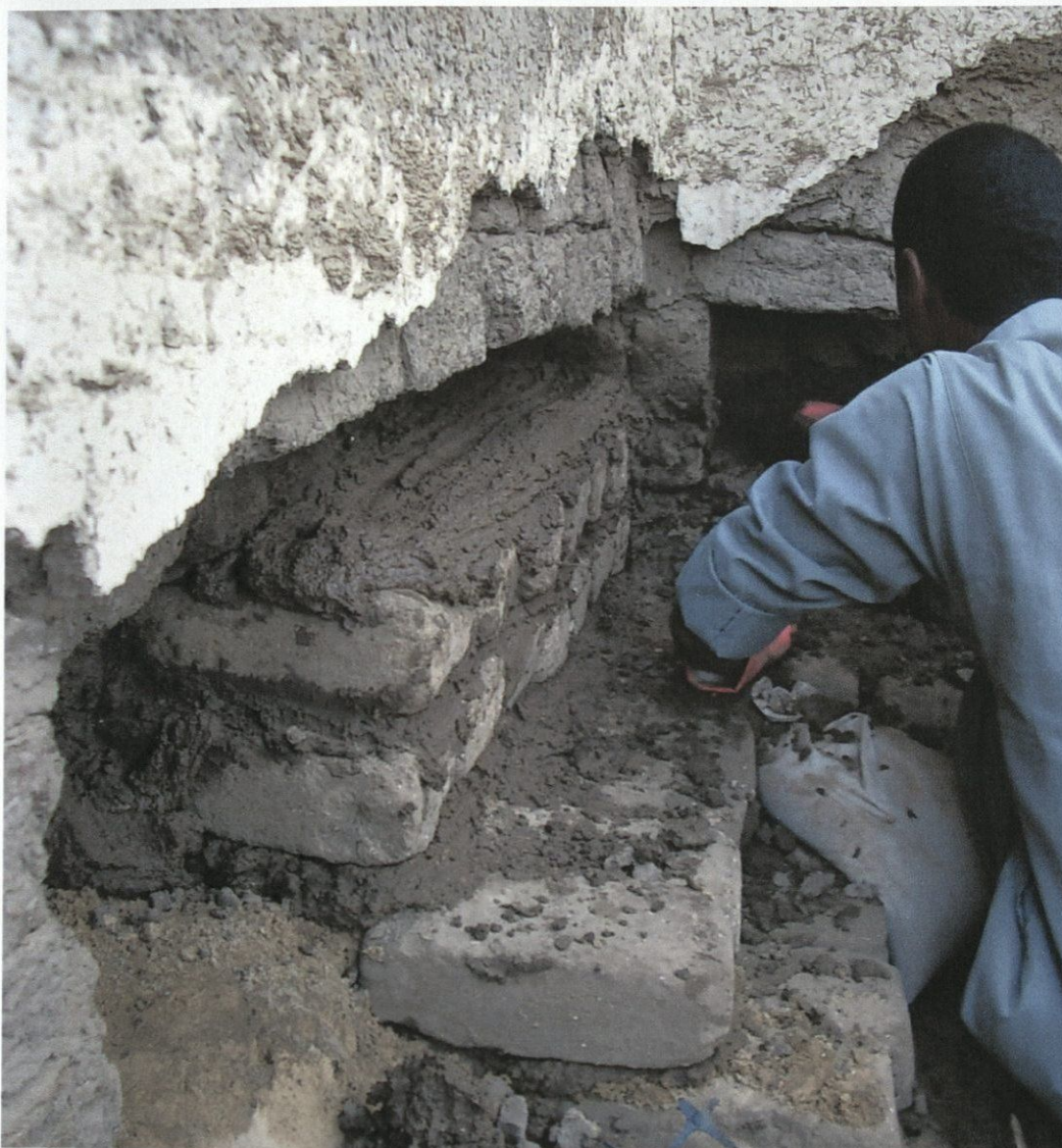
Figure 9: Mud brick masonry is being stepped back to the original wall face.
