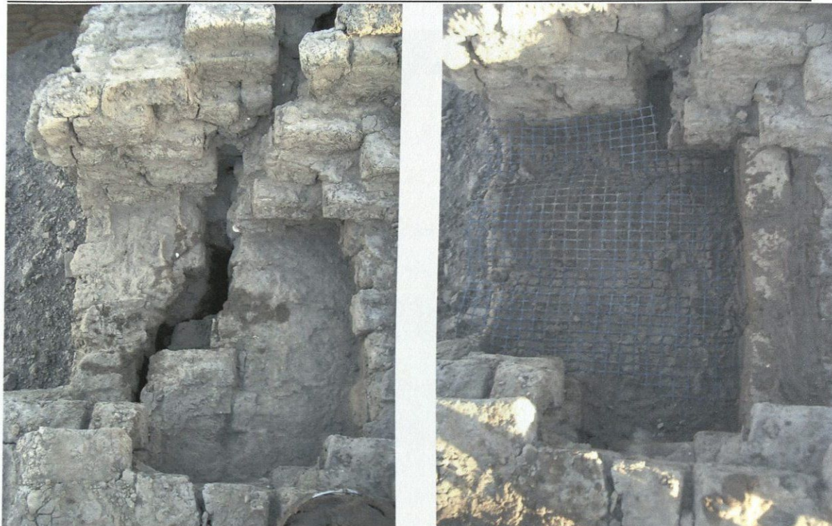
Figure 10: Detail of crack prepared for grouting and after grouting, bed mortar placed with geogrid.
