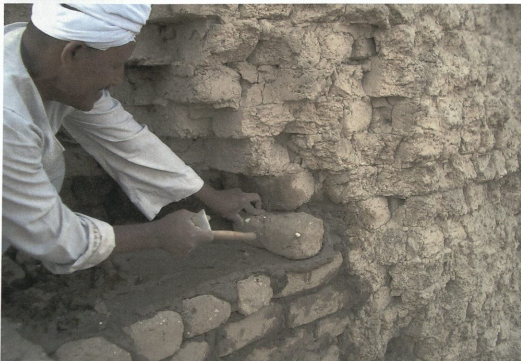
Figure 2: Integration of existing mud brick construction with new construction by the creation of a "toothing" pattern.
