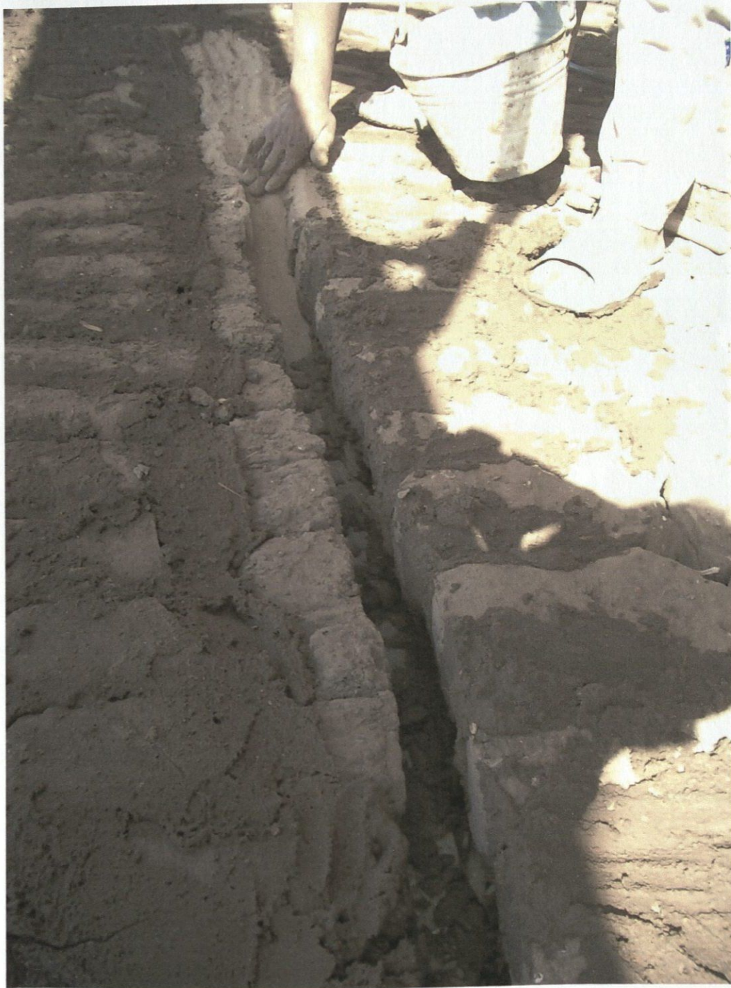
Figure 11: Sand is being added to space between mud brick and vertical plaster.
