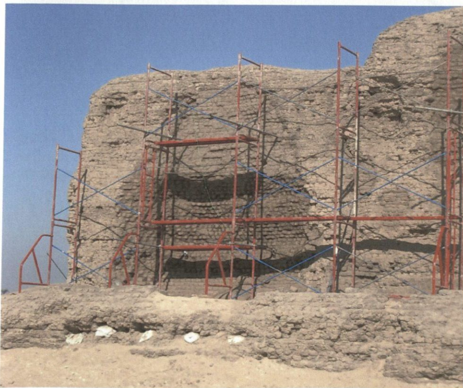
Figure 1: North cell on west wall with top half treated with mud wash to blend with original wall surface during process of a similar treatment for all the new bricks on this section
