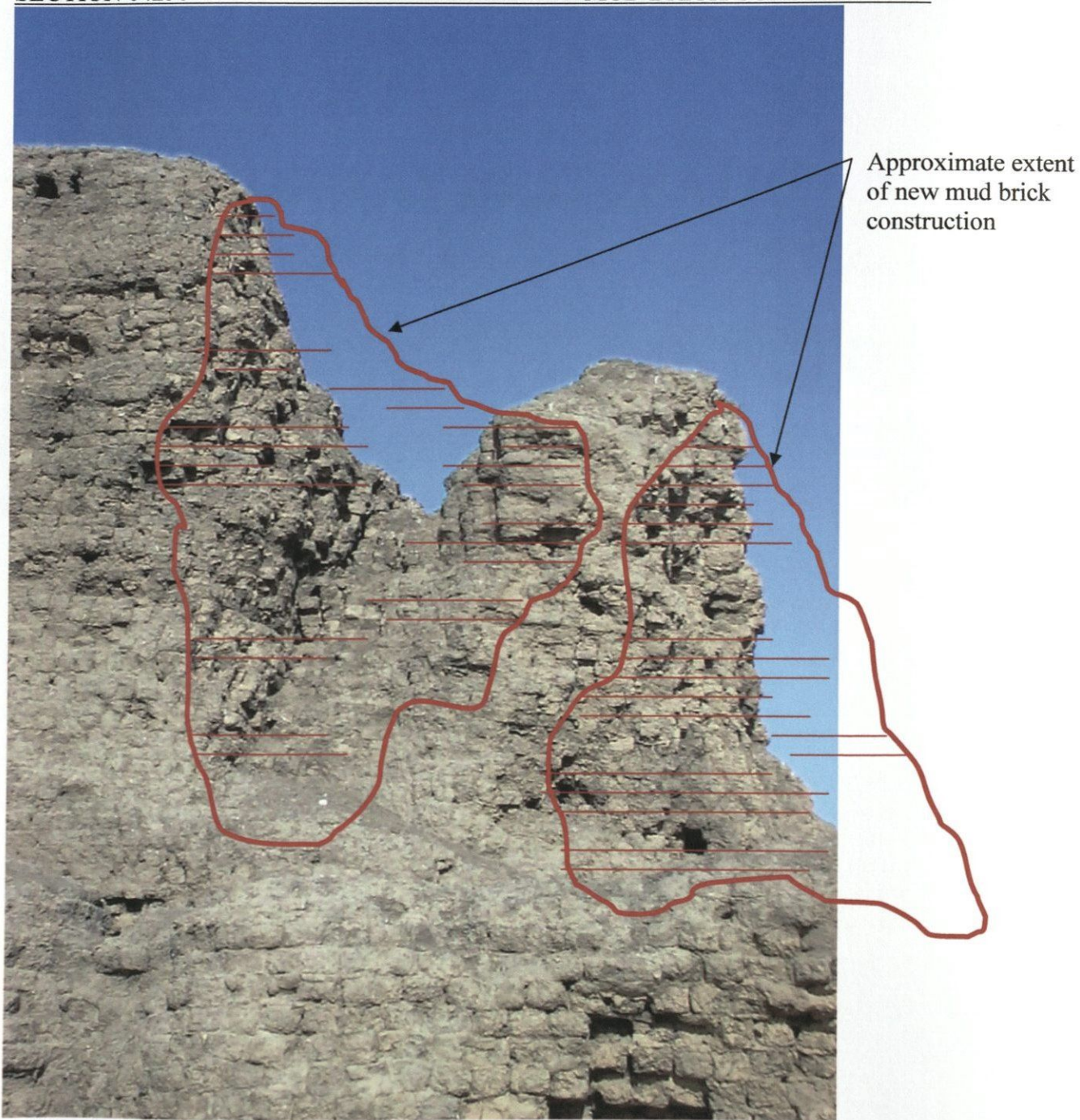
Figure 9: Detail of an area of missing wall mass at the southeast corner. The missing sections were reconstructed in 2005.
