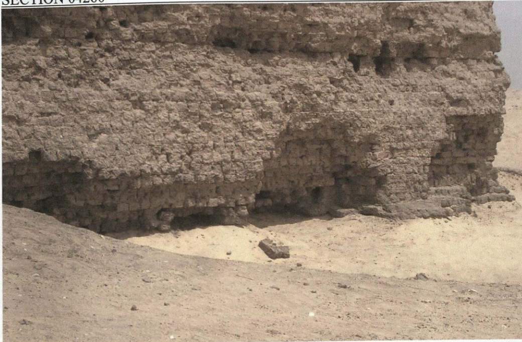
Figure 2: Another example of a wall base that will have to be stabilized. This large section of wall is at the southwest corner of the enclosure wall.
