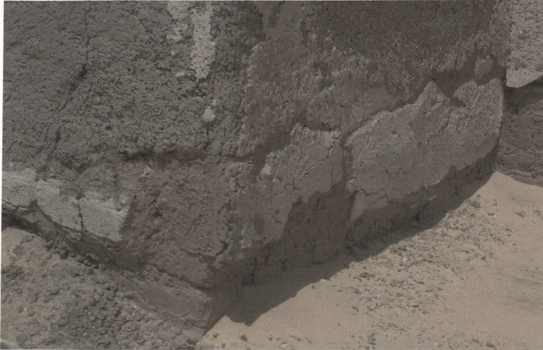
Figure 10: The reattached plaster in place after it has cured and the sand bag supports have been removed.
