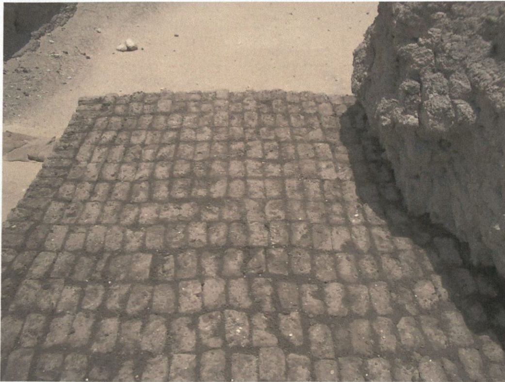
Figure 3: Comprehensive pointing of a course of mud bricks prior to the installation of horizontal reinforcement.
