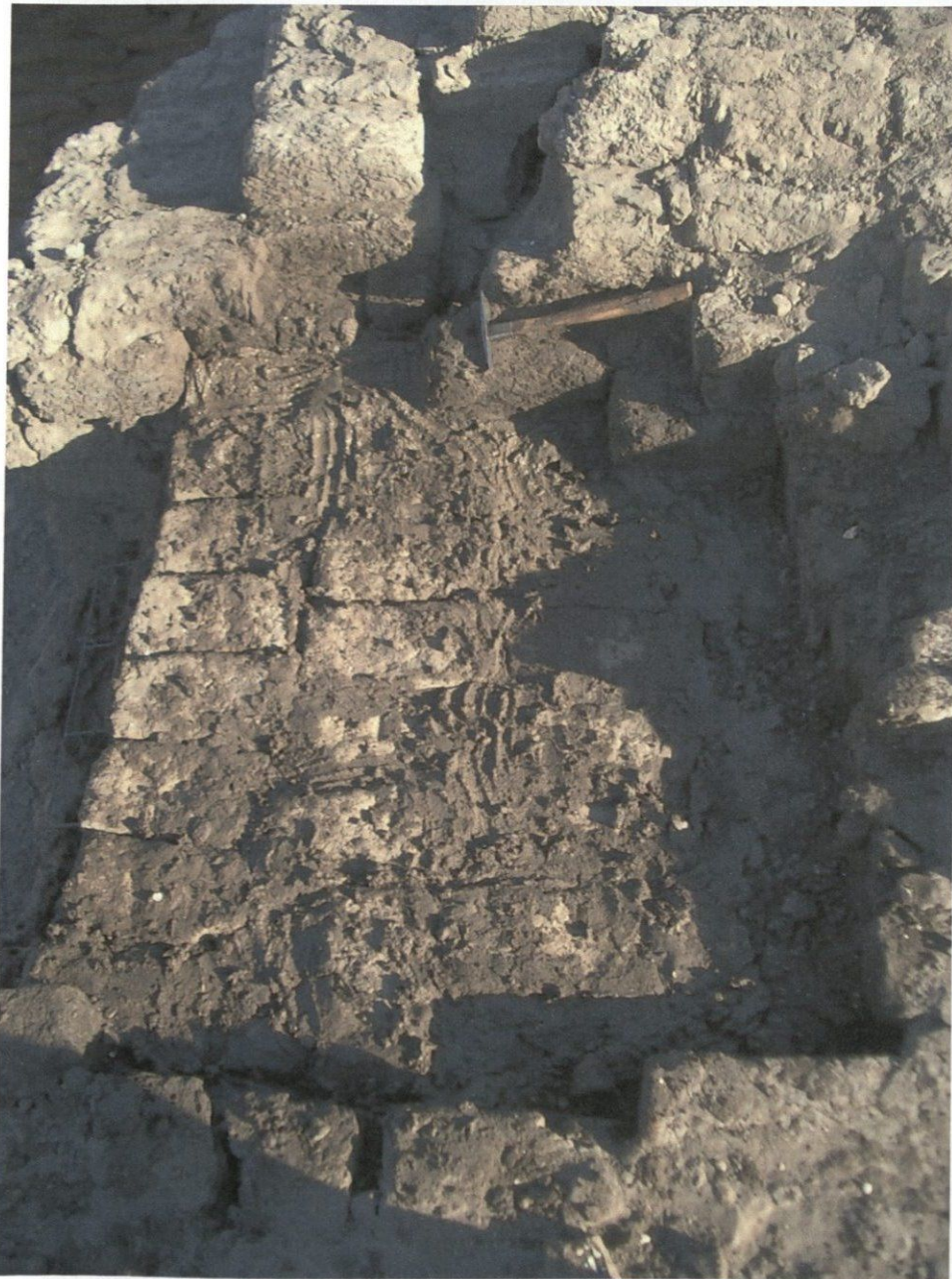
Figure 12: Void created by crack and removal of poor materials is being brought up to original top of wall.
