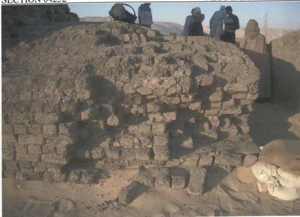
Figure 3: Detail of the base of the west side of the door showing deteriorated and missing lower wall. This part of the base had to be comprehensively stabilized by reconstructing this part of the base.
