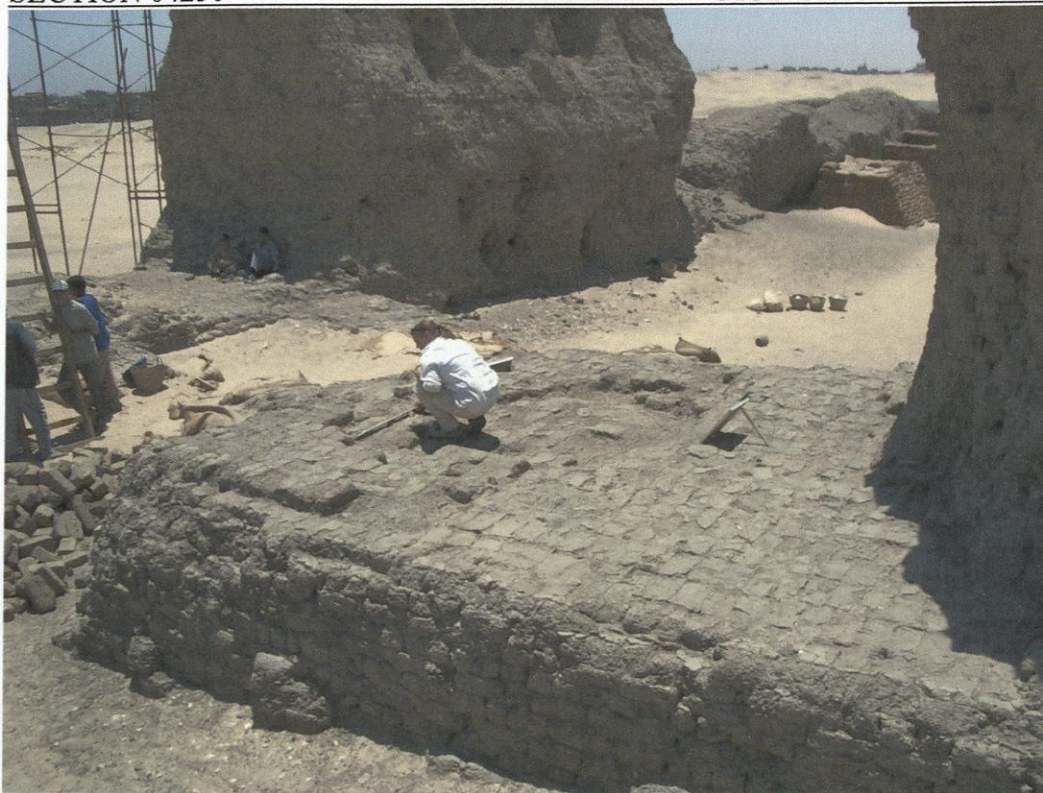
Figure 1: Preparation of mud brick base has been completed for new construction. Documentation of the base is underway.
