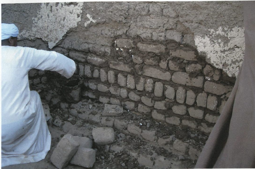
Figure 10: The wall base is being completed masonry packed and wedged in as much as possible. Note small white rocks used to reduce settlement as mortar dries.
