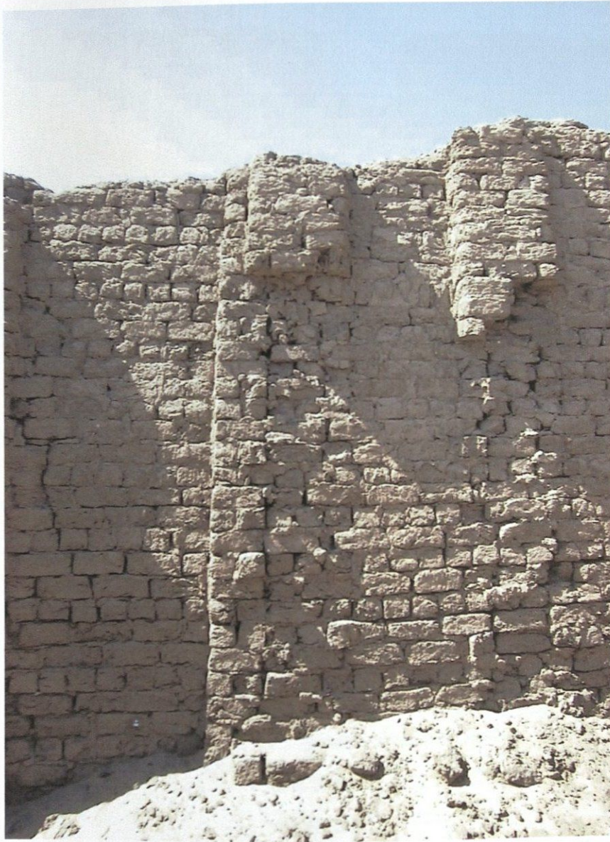
Figure 6: Deteriorated pilaster with recent fall of mud bricks and fragments.
