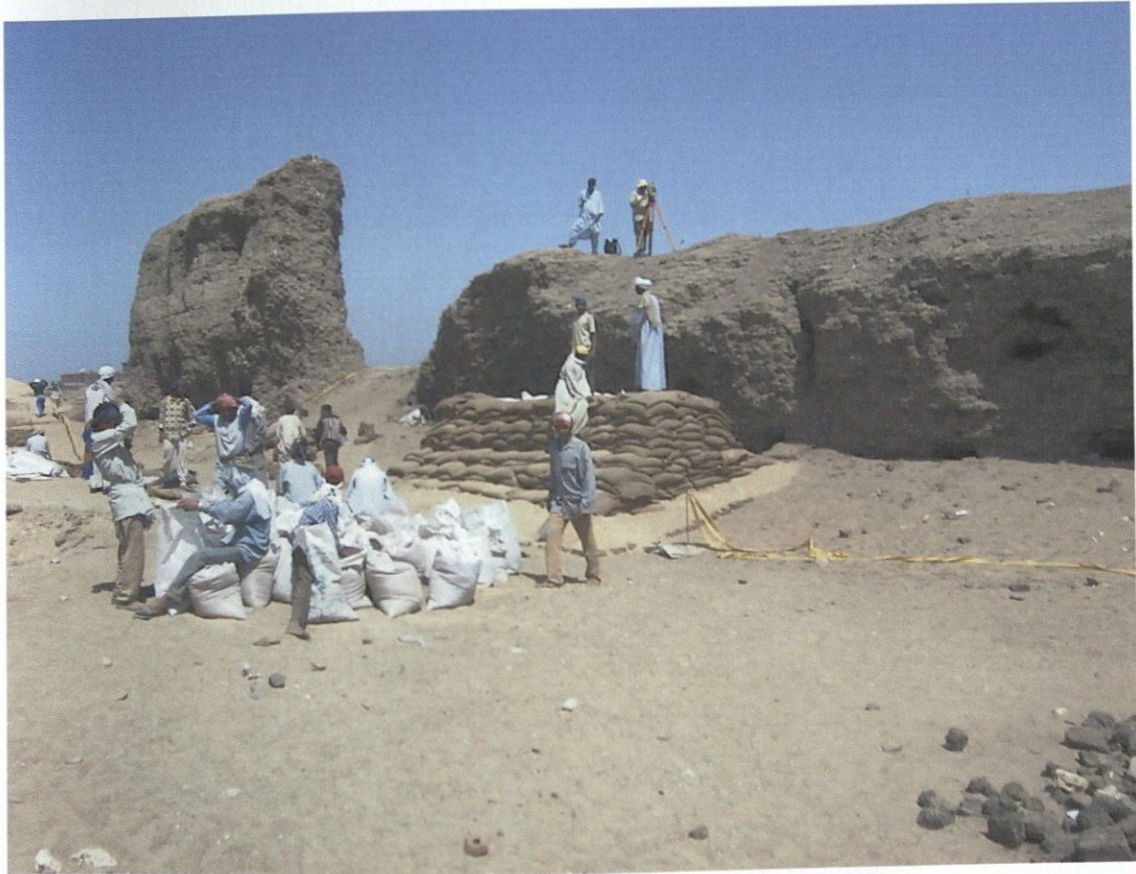
Figure 3: A sand bag buttress under construction on the west side of the East Enclosure Wall in March 2001. See Figure 4 for a detail of this same condition.
