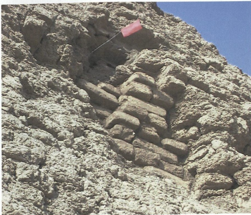
Figure 7: Detail from below of the repair to the West Enclosure Wall. Note repair is corbelled to support mud brick above.
