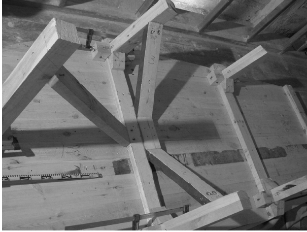
Fig. 3. Underside of platform after cutting to the contour of the lid outline, showing placement of supports.
