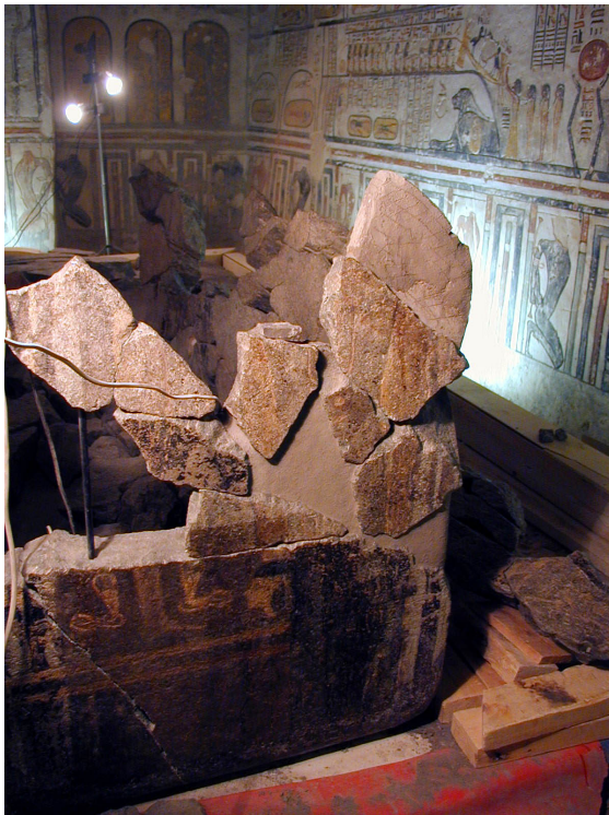
View showing the filling of missed areas by hydraulic lime and stone powder
