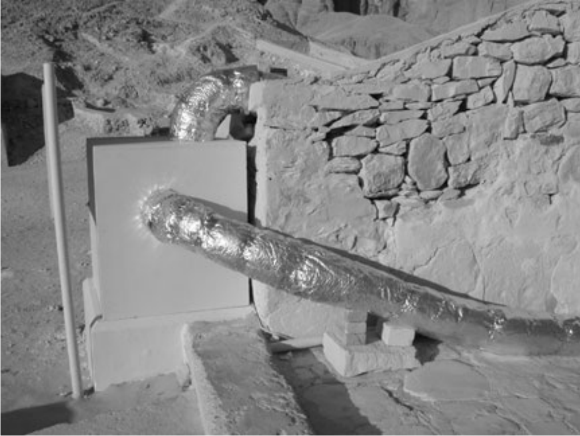
Figure 3. Detail of foil-coated insulation covering exterior tubing.
