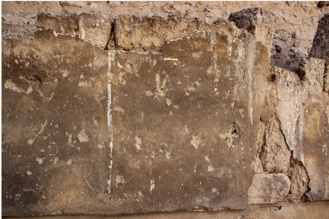
Bird lime and sooty deposits
