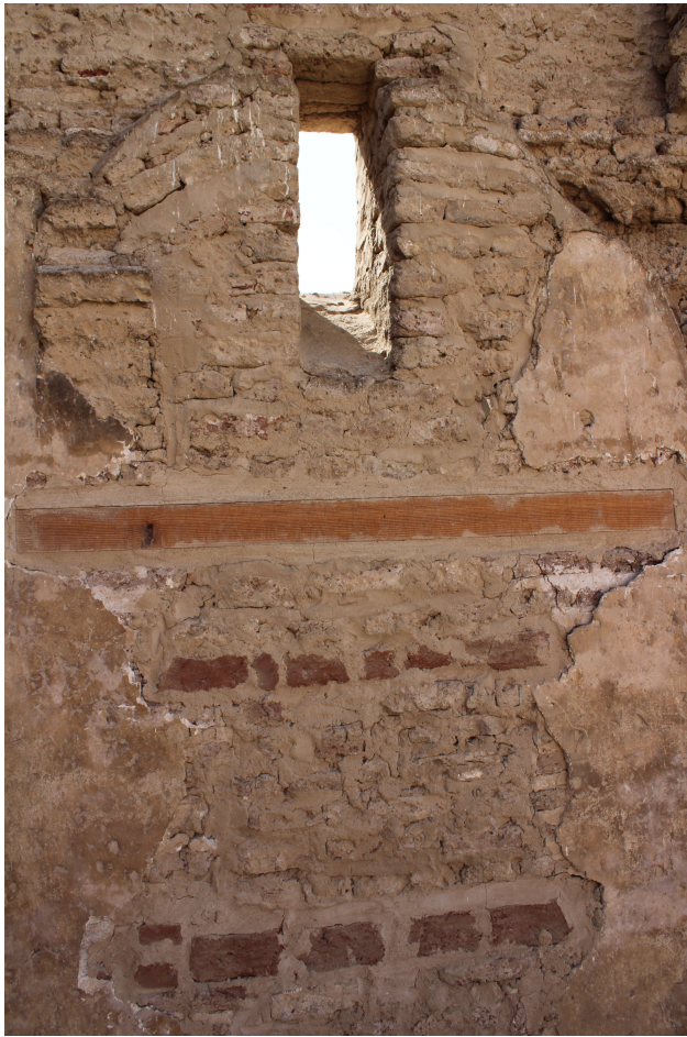
Detail of one of the wooden beams and associated materials used in the stabilisation of the section of wall
