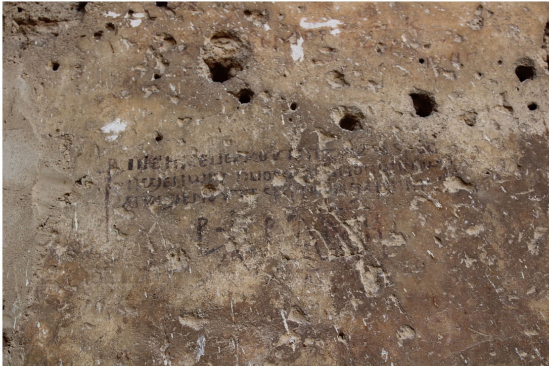
Cement repair to the left of the dark red text, at the junction with the south wall
