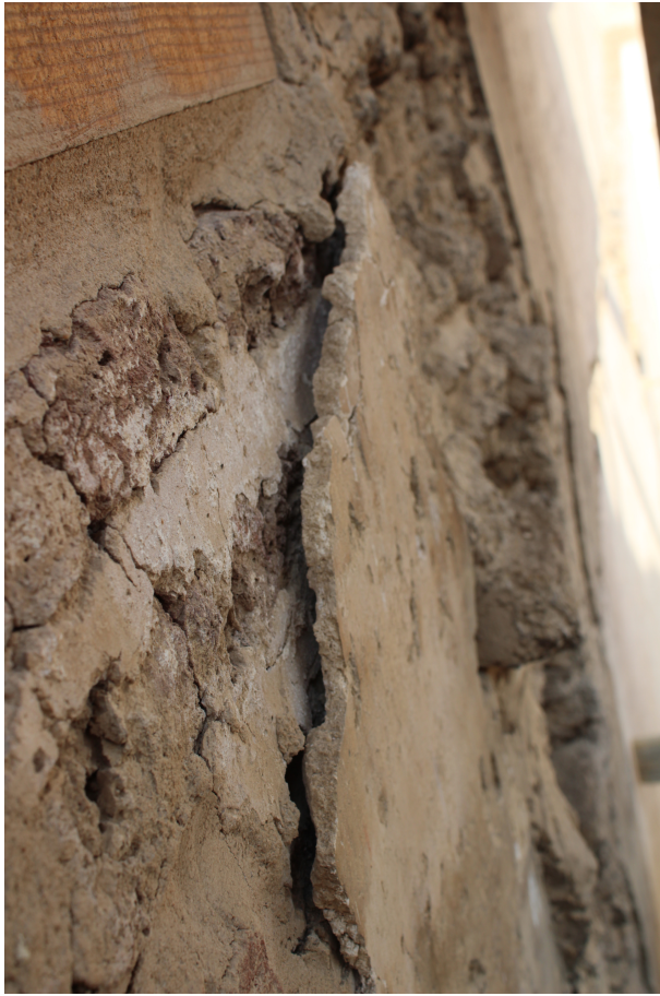
Detail of detaching plaster
