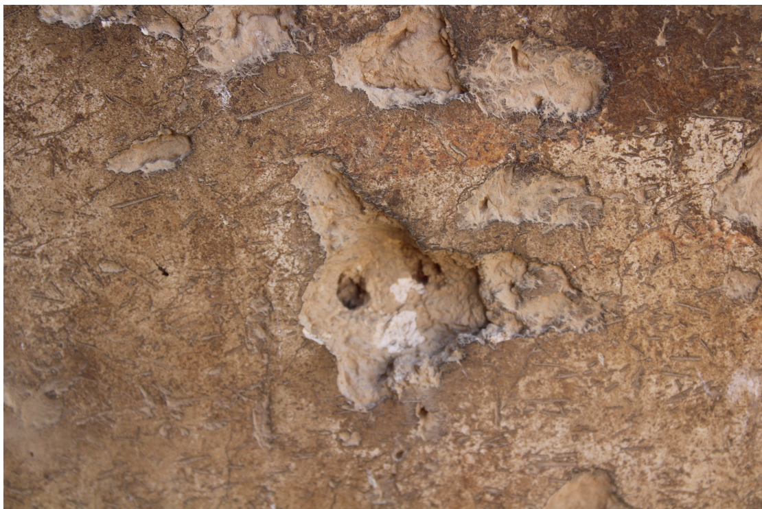
Small holes and losses and masonry bee damage
