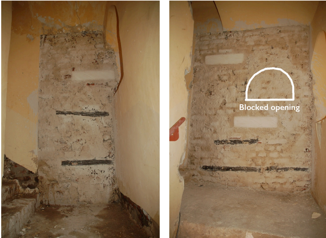
Timber and stone stitches in the south wall of the stair at lower (left) and upper (right) levels
