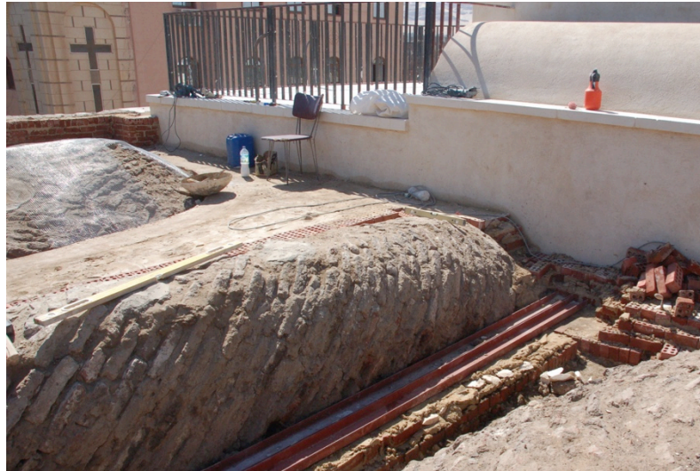
View from northeast of elliptical vault showing location of new steel reinforcement during installation
