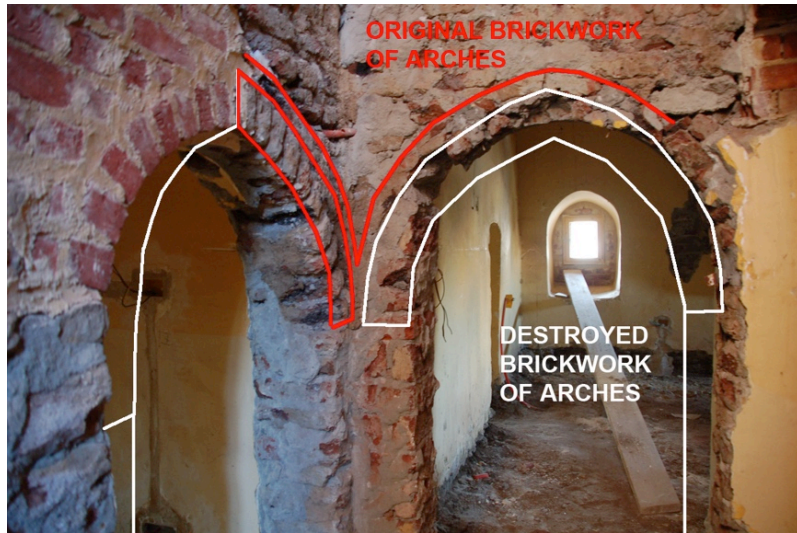
Diagnostic view of entrances to first floor rooms from staircase after removal of cement render
