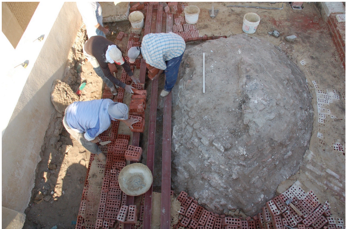
View from west of three new steel beams during installation on north side of north dome to take loading off weakened section of dome
