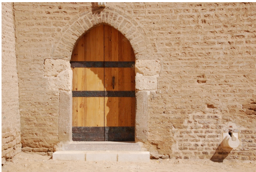
Installation of new granite threshold (top); new pitch pine doors after installation (bottom)
