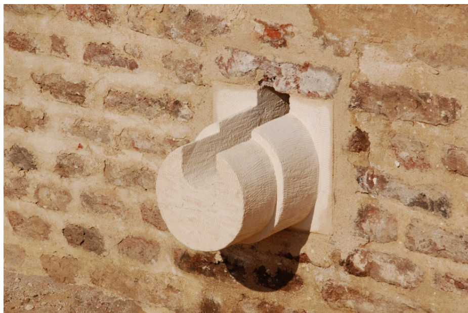
New limestone drainage spout on line of existing water channel embedded in the west wall of the tower
