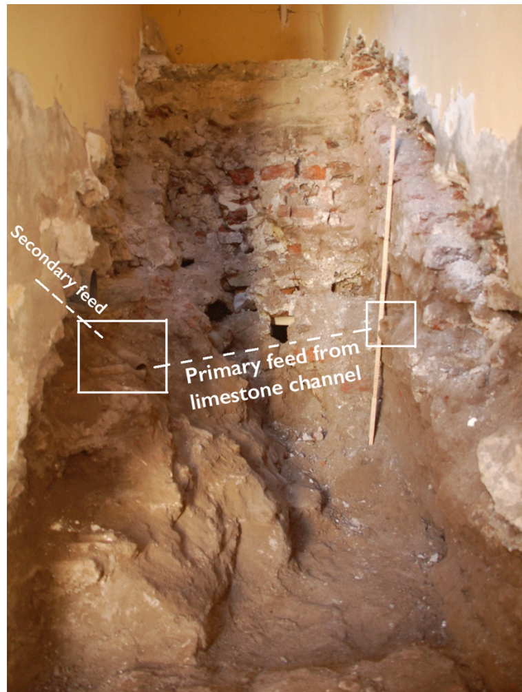
View of location of interlocking lines of ceramic pipes under the tower staircase looking south
