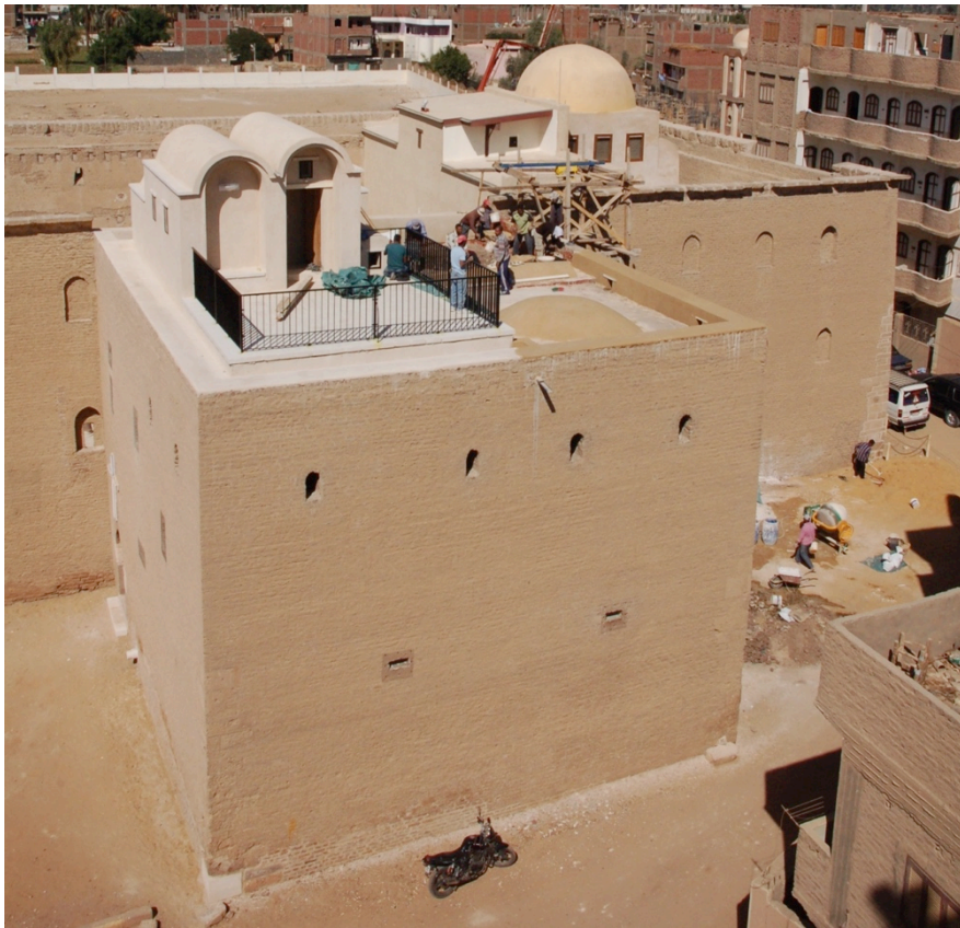
Views of the roof of the tower from the south before (top) and during (bottom) interventions
