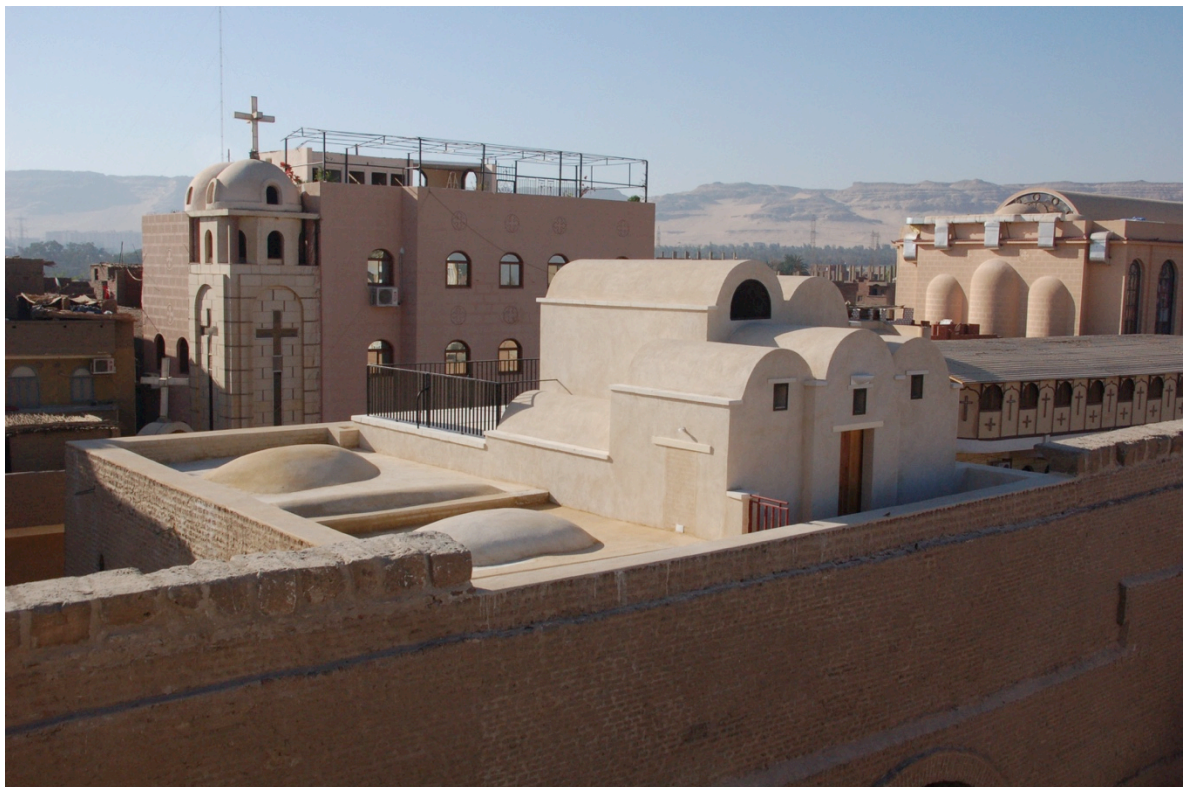
View of completed intervention on roof from northeast showing lower vaults plastered to fall and new staircase structure to right
