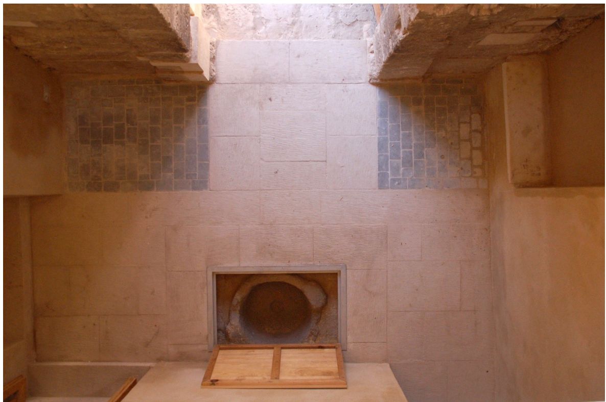
Condition of entrance area seen from above after treatment with trapdoor over granite basin
