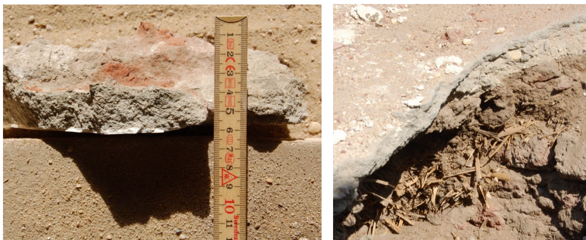
Section of typical 5cm thick cement render from the interior of the tower (left) and cement renders over organic fill on roof (right)
