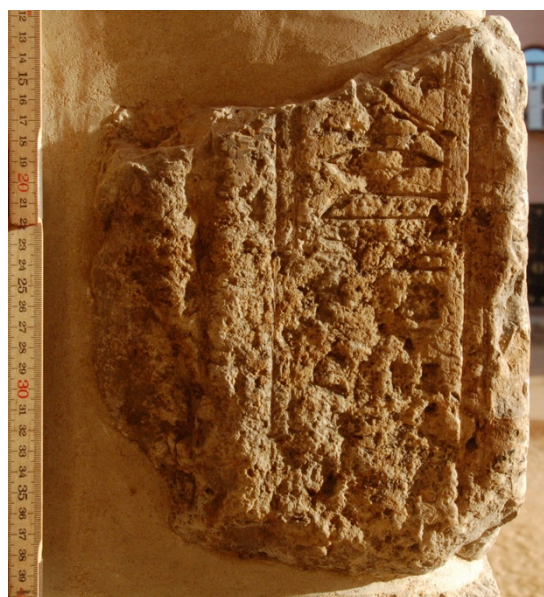
Inscribed block from south jamb of main entrance door to tower after cleaning
