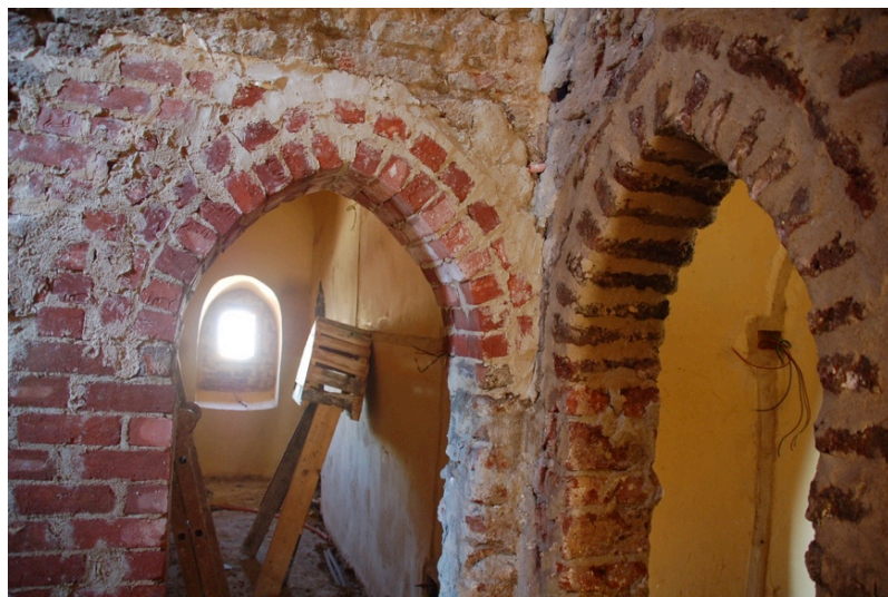
The doors to the first floor after masonry consolidation following traces of the original arches
