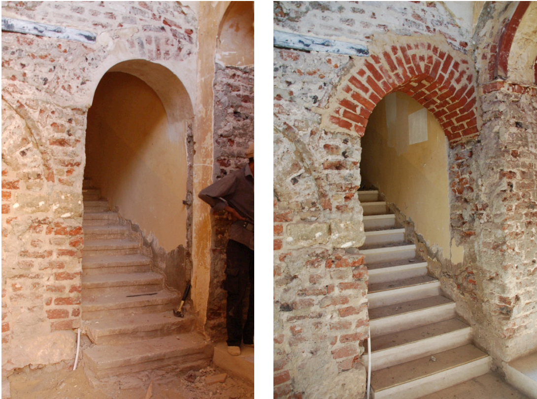
Arch over first flight of staircase before (left) and after (right) rebuilding
