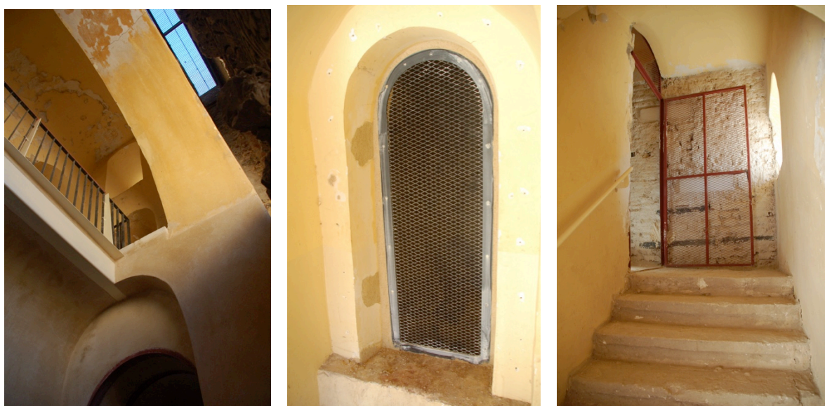
General view of balcony looking up (left); typical steel frame window with bird mesh deterrent (center) and steel gate on staircase with bird mesh (right)
