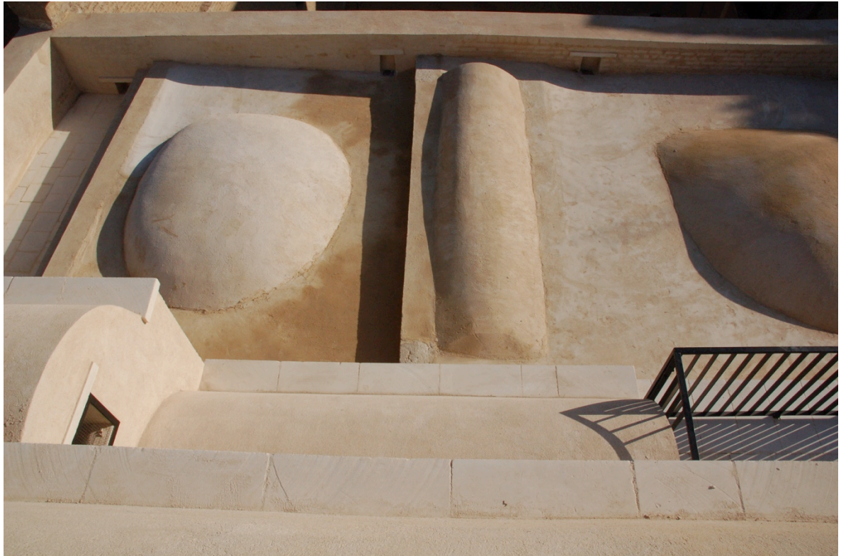
View of completed intervention on lower area of roof showing vaults plastered to fall to new external rainwater spouts
