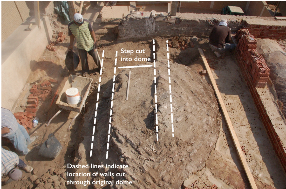
Diagnostic view of north dome showing secondary damage
