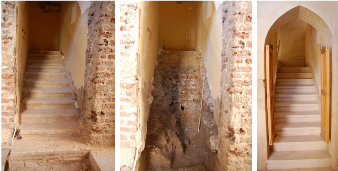
First flight of staircase before (left), during (center) and after (right) reconstruction
