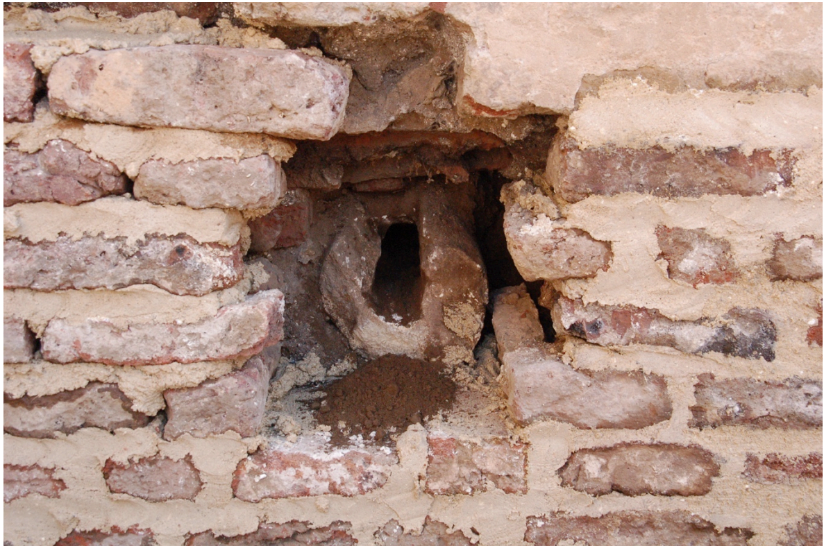
Limestone drainage channel in west face of tower
