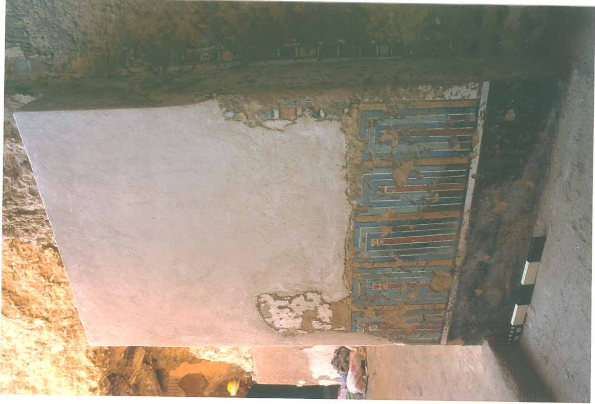
B: South reveal after repairs and cleaning by Parandowska and Warris (photo: F. Dzikowski no. EG 2 S 254 02).
