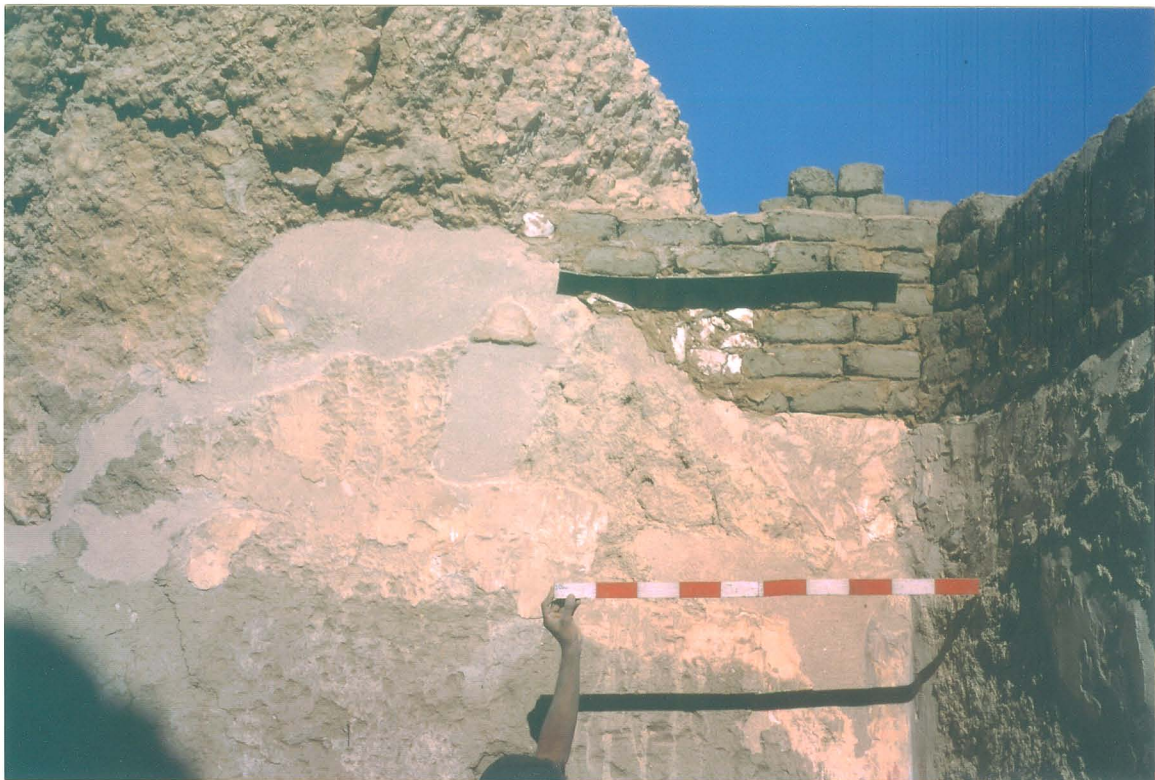
B: Inner Hall, north end, showing installation of flashing to prevent entry of rainwater. Photo: E.C. Brock, no. EG 4 S 253 02)
