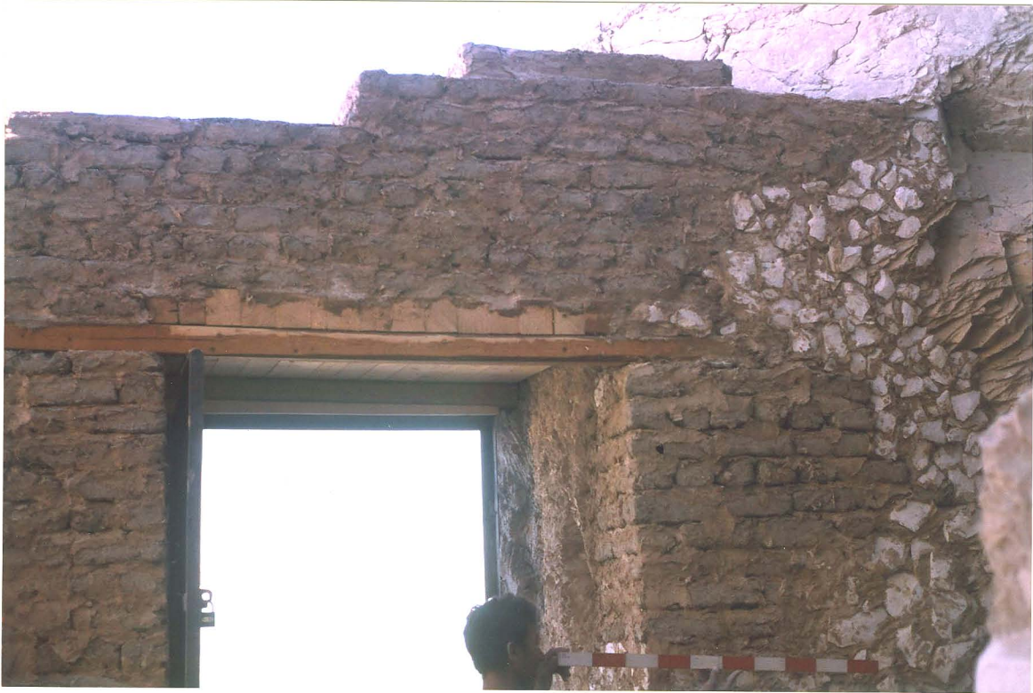
A: View of new lintel made of mud brick looking east (photo, E.C. Brock, no. EG 19 S 253 02).
